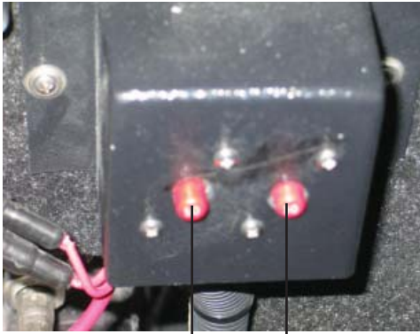
50 AMP MAIN BREAKER
