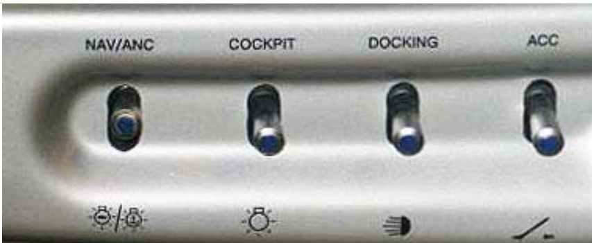
Typical Port Switch Panel
