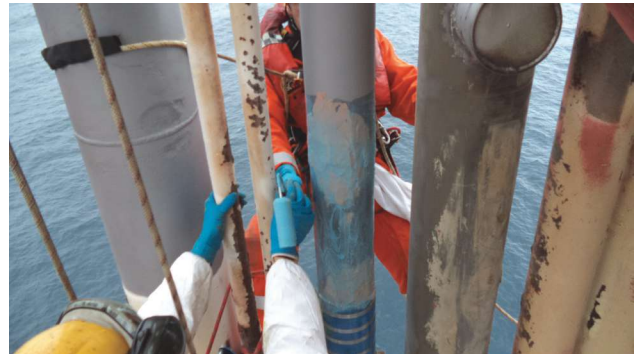
Using rollers to apply adhesive, the installation team places and secures the composite sleeves. (Source: Clock Spring)
