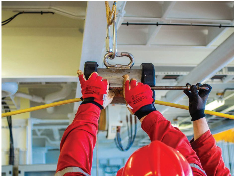
Figure 4. Gun mechanic securing tow cable to sliding collar on ceiling.
