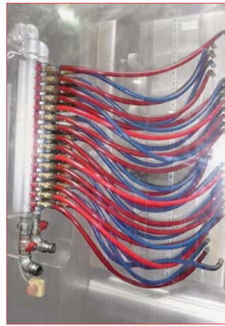
DME cooling manifold
