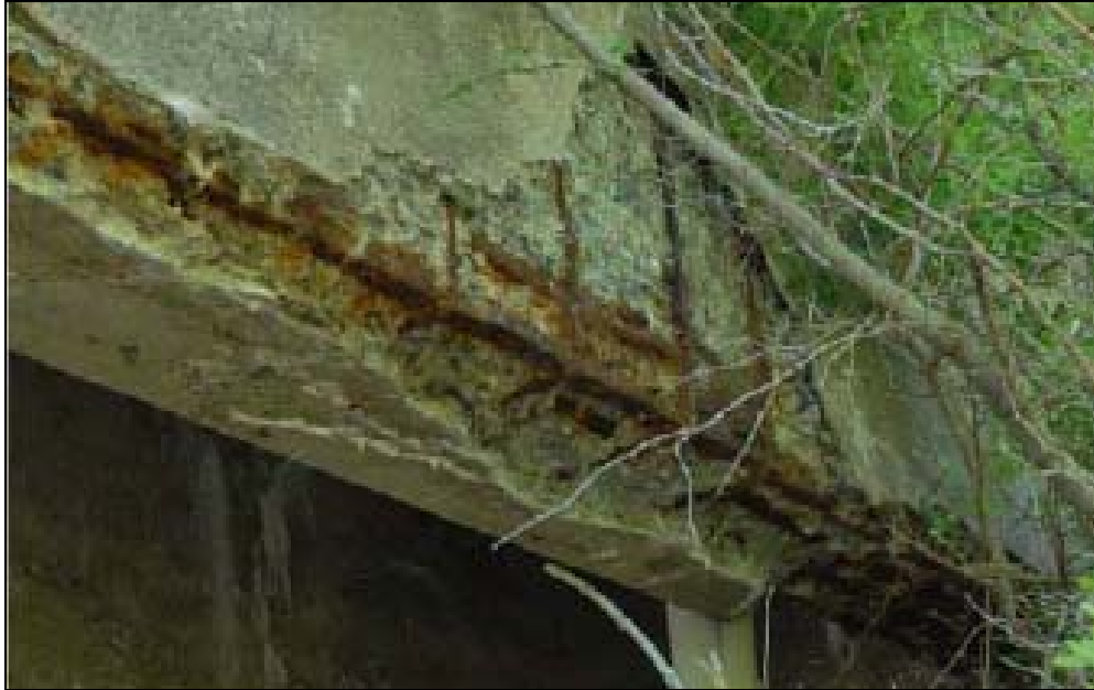
Figure 82b: Corroded girder of a PennDOT bridge
