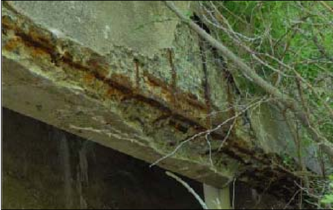
Figure 122 Figure Corroded exterior girder of PennDOT Bridge #49-4012-0250-1032
