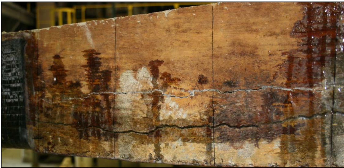
Figure 81b: New crack running parallel to injection-repaired crack in beam G-9
