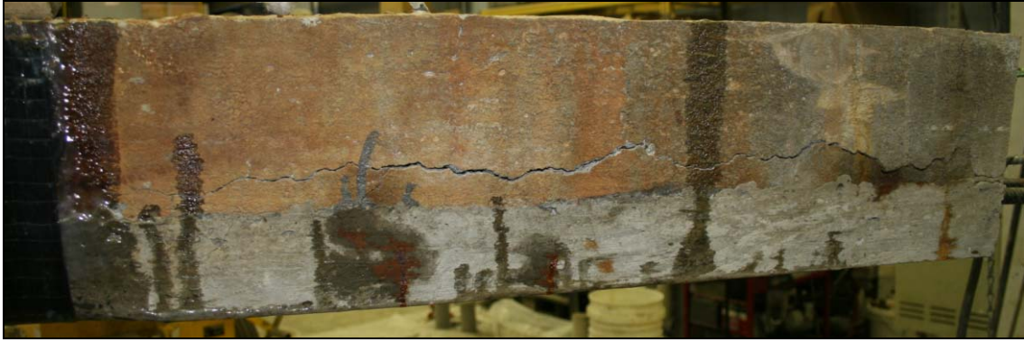
Figure 81a: Cracks in beam G-8 within the old concrete running parallel to patched concrete interface
