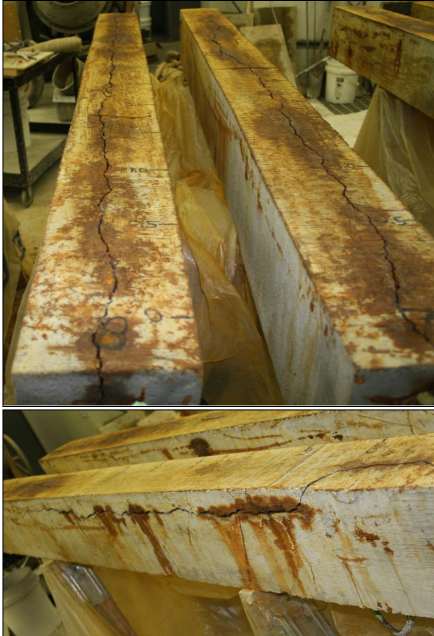
Figure 101: Typical deterioration of Part II beams prior to repair
