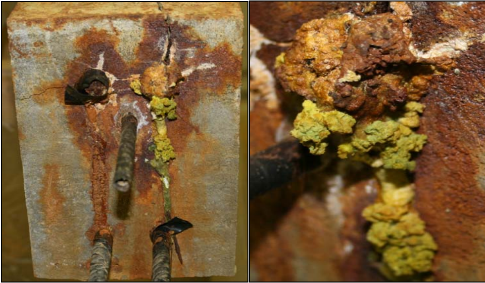
Figure 102: Typical deterioration of Part II beams prior to repair.
