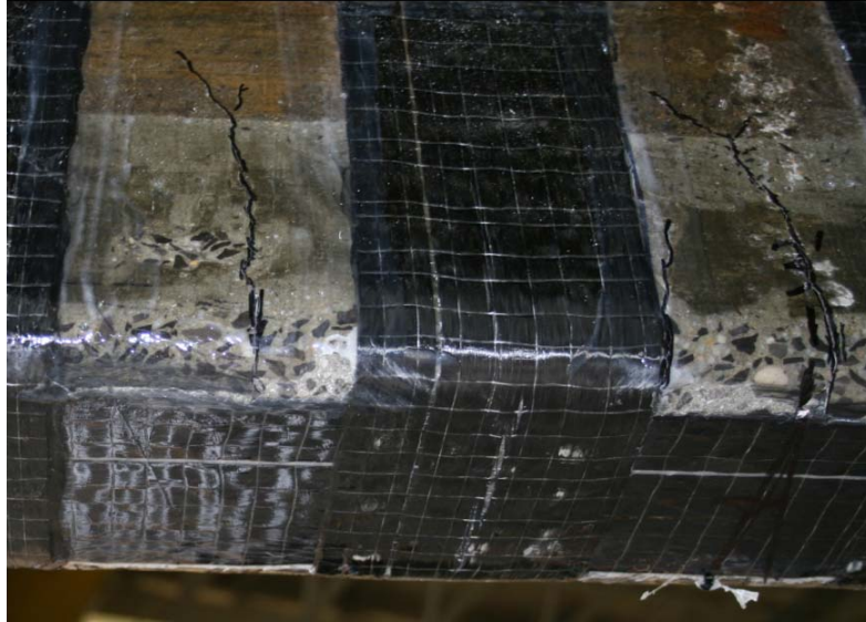
Figure 124: Composite action between old and new concrete on Part II beams as evidenced by cracking continuity across interface
