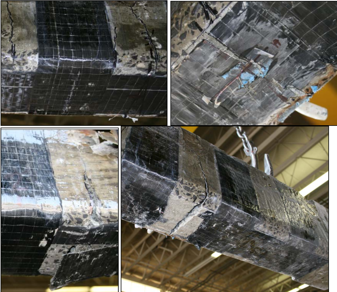
Figure 119: Photos of non-fatigued Part II beams repaired using Wrapping Scheme 3 after failure
