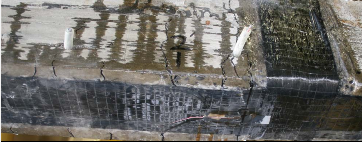
Figure 117: Photos of non-fatigued Part II beams repaired using Wrapping Scheme 2 after failure
