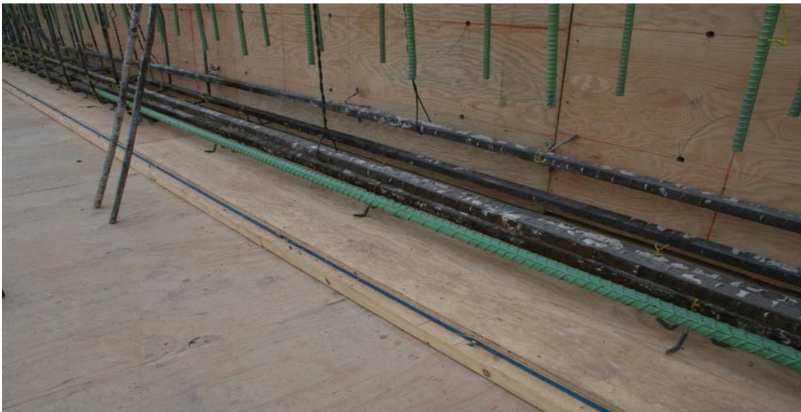
Figure 3: Central Portion of Beam 6 with Two Missing Bars in the Top Layer of Tension Steel
