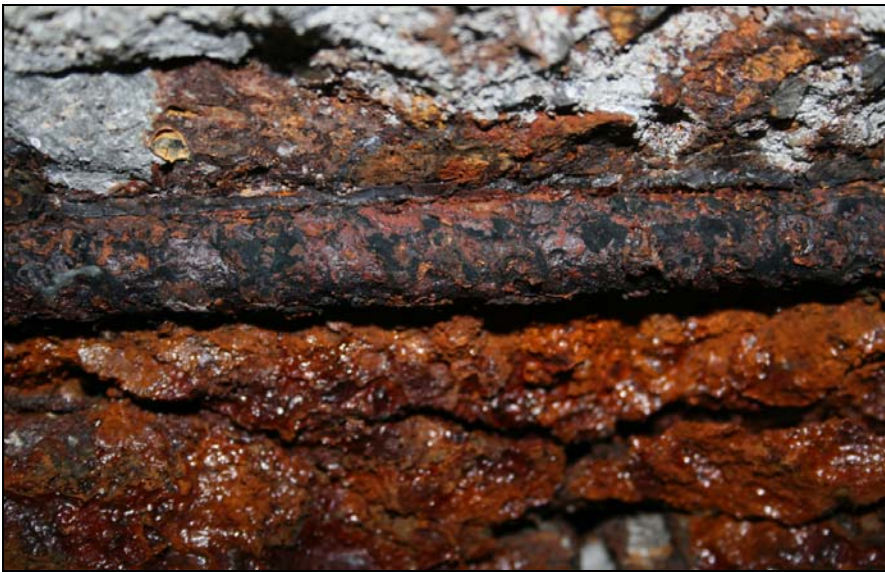
Figure 103: Corrosion observed in Beam II-3 after cover delamination
