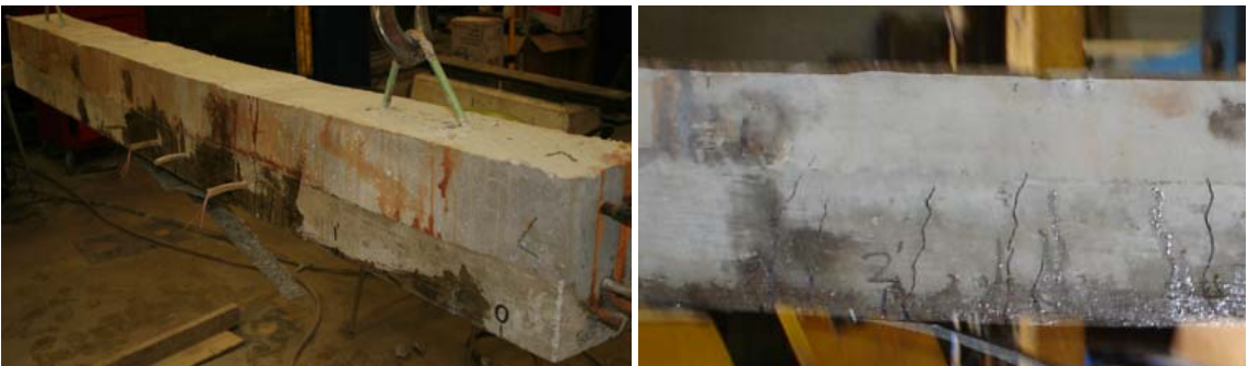
Figure 116: Photos of fatigued Part II beams repaired using Wrapping Scheme 1 after failure
