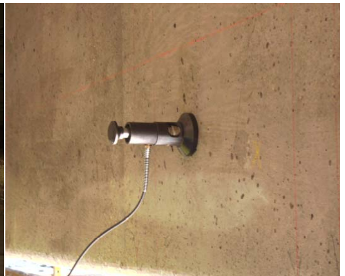
Figure 8: Tension Test of Portion of Patch Material using the Portable Adhesion Tester
