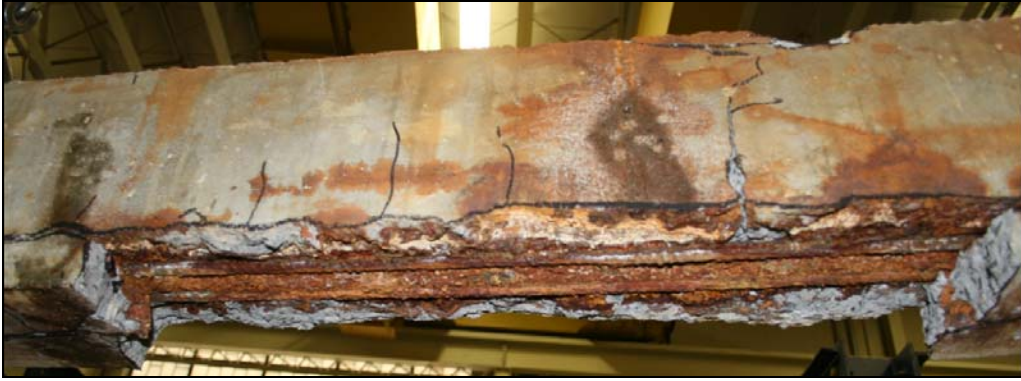
Figure 82a: Corroded beam sample
