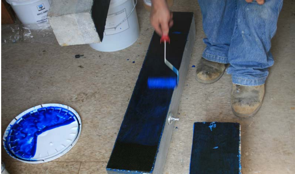
Figure 14: Installation of FRP using to Roller to Fully Impregnate the FRP with the Resin
