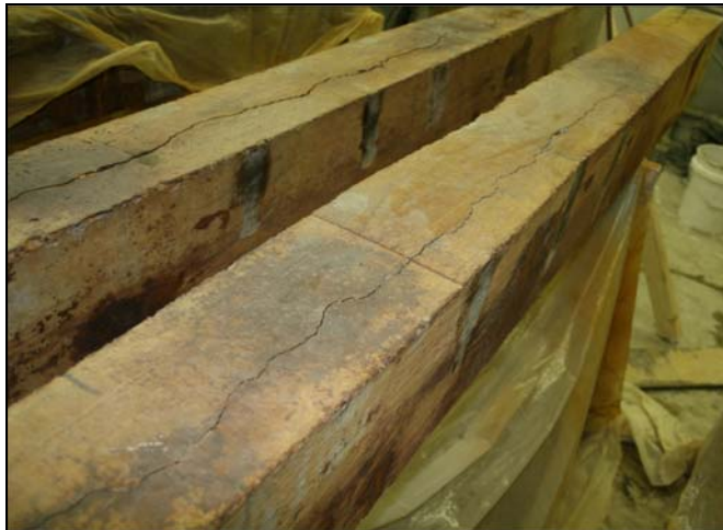
Figure 80: Typical extent of deterioration observed after initial corrosion
