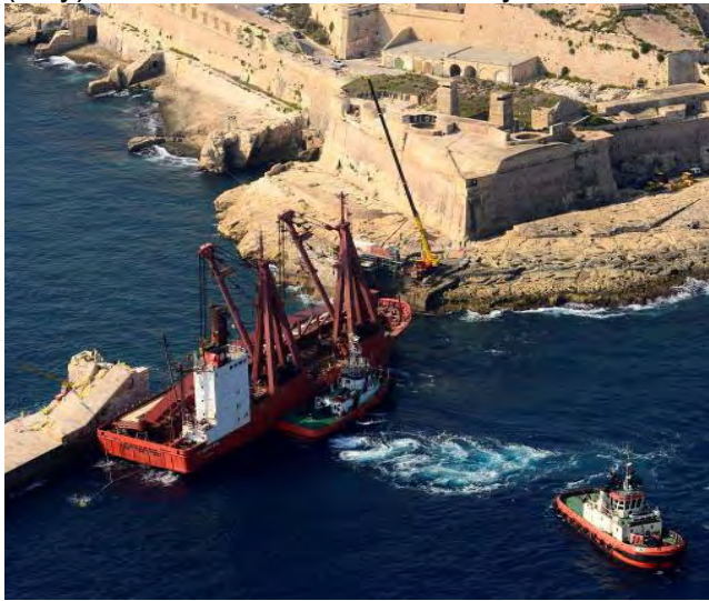
The Storman Asia is erecting the bridge over the local breakwater in Valletta (Malta), October 2011 © Airphotomalta / Marinetrain
