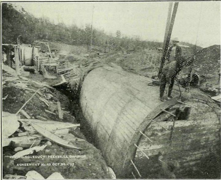
View of Pipe on Peekskill Division.
