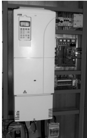
Fig. 2. The inverter ACS 800 and the controller NI sbRIO 9606
