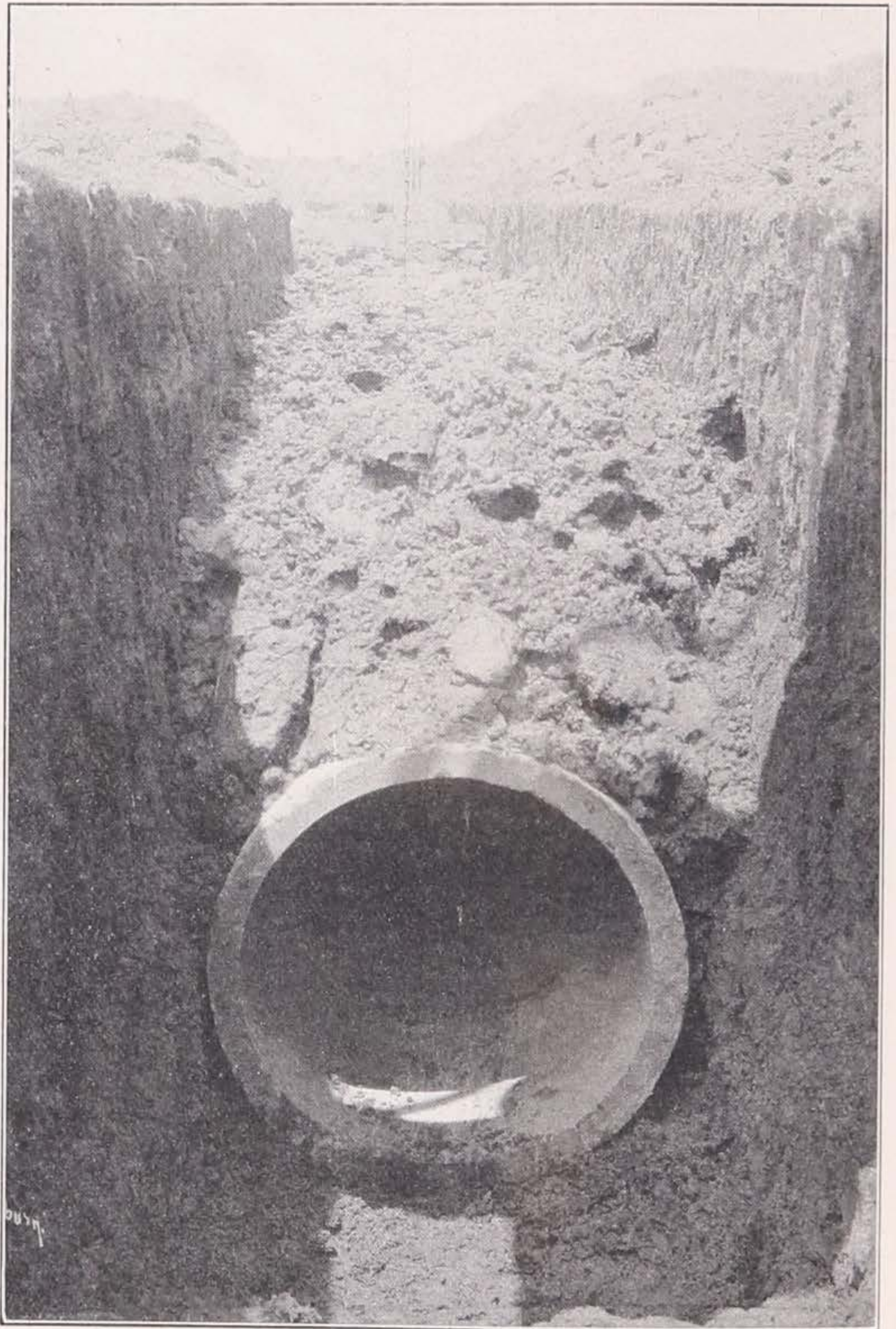
Fig. 22. Photograph Showing Typical Actual Field Conditions of Bedding and Loading of Pipes in Ditches.
