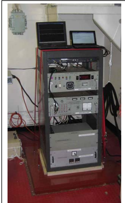
Figure 1-22. BGM-3 Electronics and logging computers installed in Louis Gravimeter Compartment # 615.
