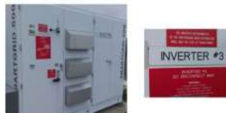
Typical Inverter Signage /NFPA
