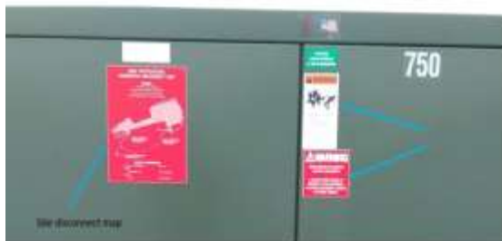
Typical Transformer Signage/ NFPA
