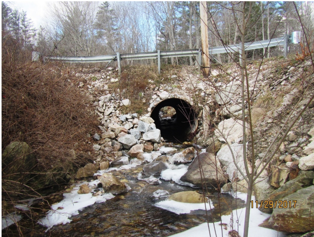
Figure 3.3: Large stones observed at the outlet of the culvert. [Inspection photo dated 2017]
