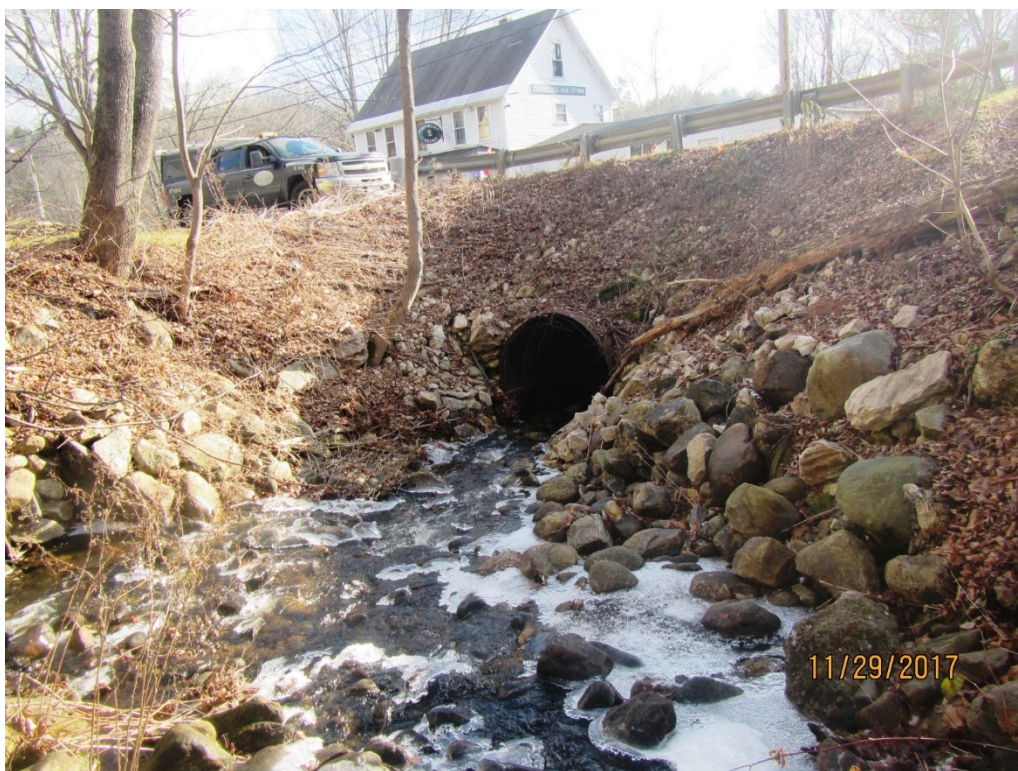
Figure 3.2: Large stones at the inlet of the culvert. [Inspection photo dated 2017]
