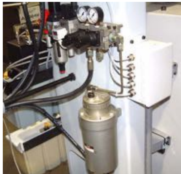
Filter Regulator Package (Located on Barfeeder)
