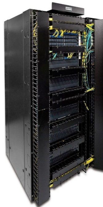
patch location rack
