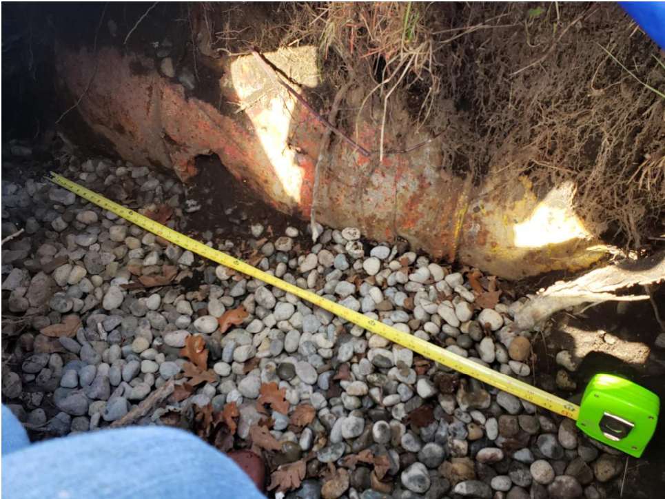
Fig. 5: Exposed barrel(s) located in the ground behind the lab.
