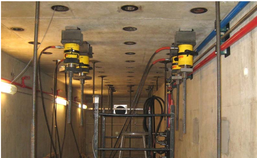
Figure 3.11 Hydraulic rams arrangement below the strong floor
