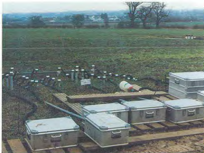
Figure 16 Installation of Pressure Transducer Tensiometers (PTTs) around a mole drain at Wytham Farm, Oxford
