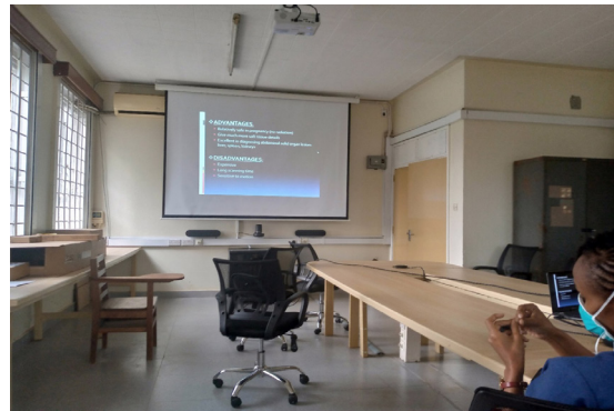
Department of Anaesthesia classroom was renovated into a virtual learning multipurpose smart classroom for masters' students
