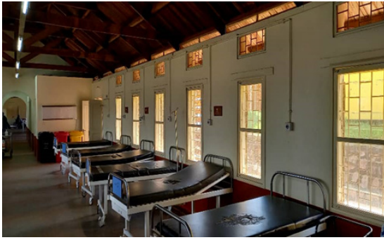
A central line for oxygen supply to beds in Ward 7 added to support patients after operation.
