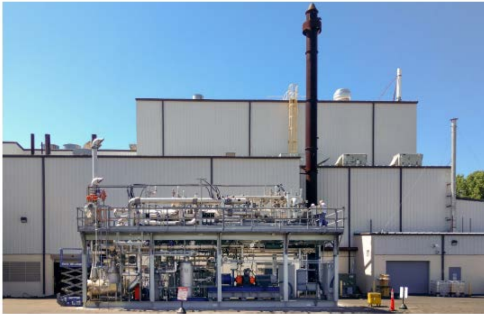
Figure 8: MTR skids installed at B&W's SBS-II research facility
