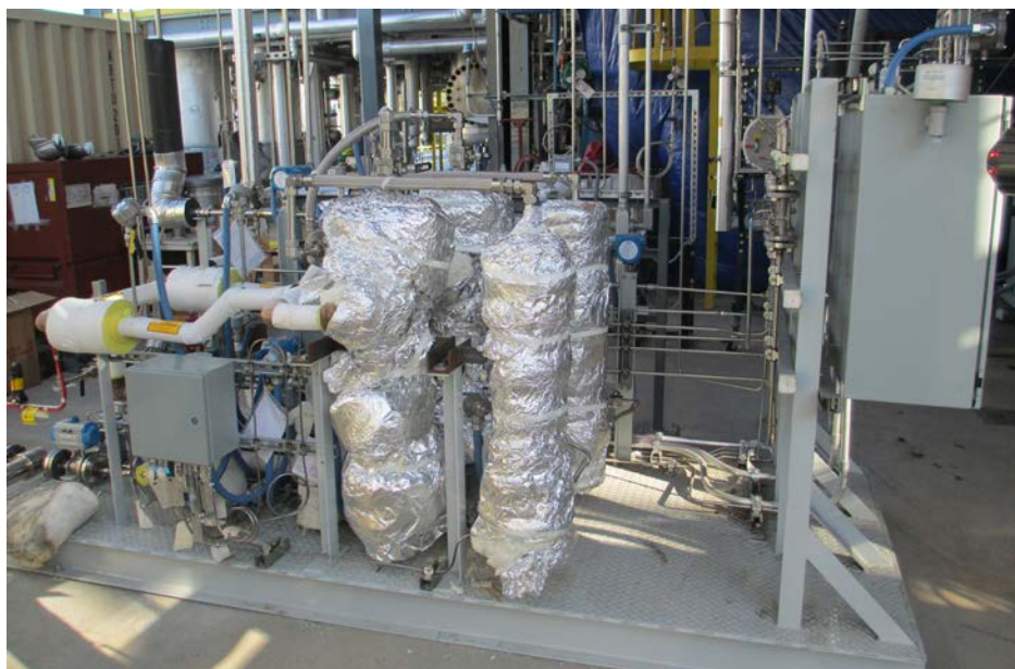
Figure 5: Photograph of the PBI skid installed at NCCC in March 2017
