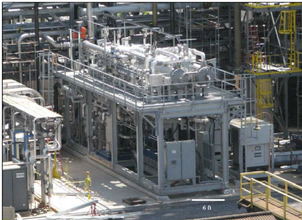
Figure 3: 20-tpd small pilot system installed at NCCC
