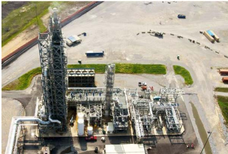
Figure 1: KM CDRProcess™ at Plant Barry
