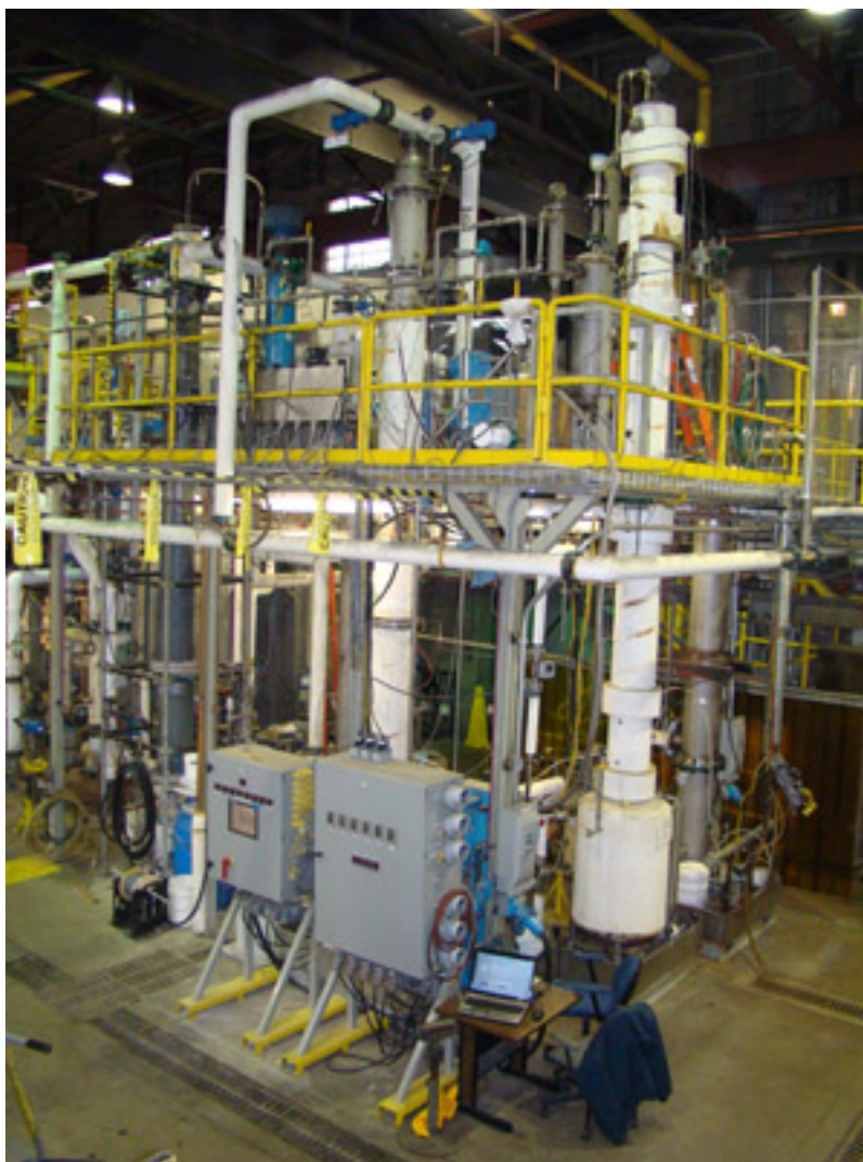
Figure 1: UNDEERC post-combustion CO 2 capture test facility
