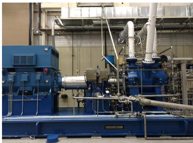
Figure 4. Installed Dresser-Rand Datum Compressor Package
