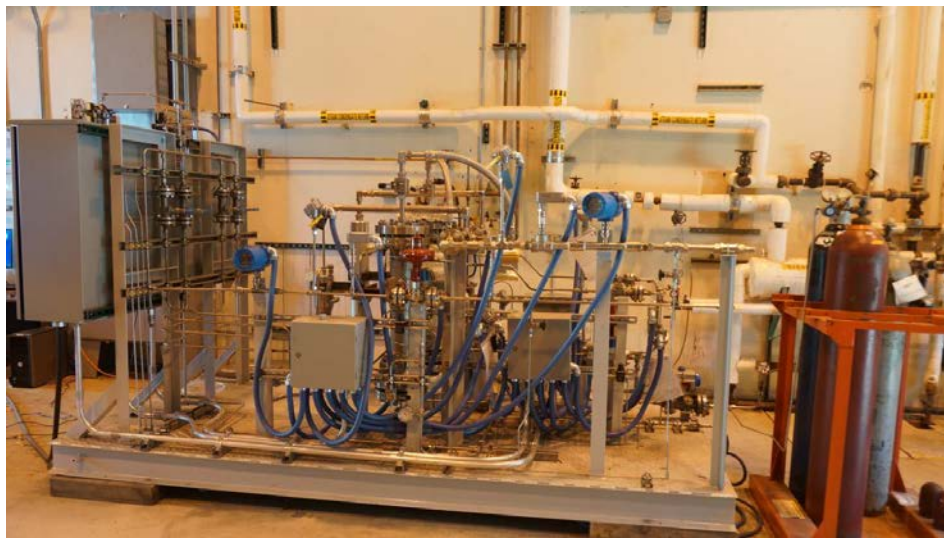
Figure 4: Photograph of the PBI skid in October 2016
