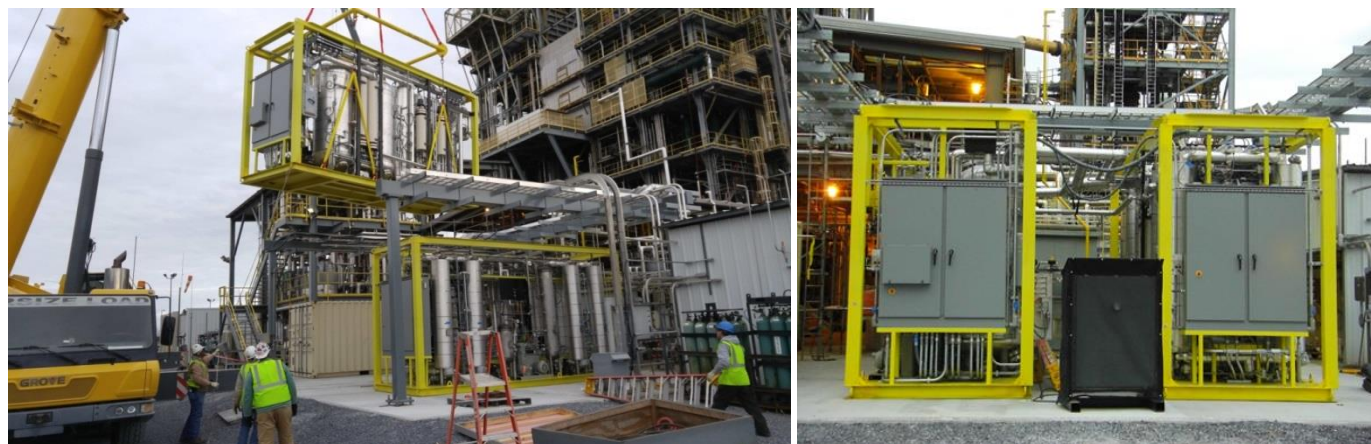
Figure 4: TDA's 0.1-MW e pilot unit installed in the test pad at NCCC (Wilsonville, AL)
