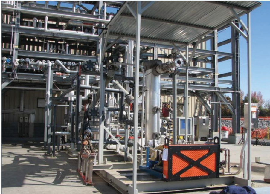
Figure 2: Membrane skid used for 1-tpd bench-scale slipstream testing at NCCC
