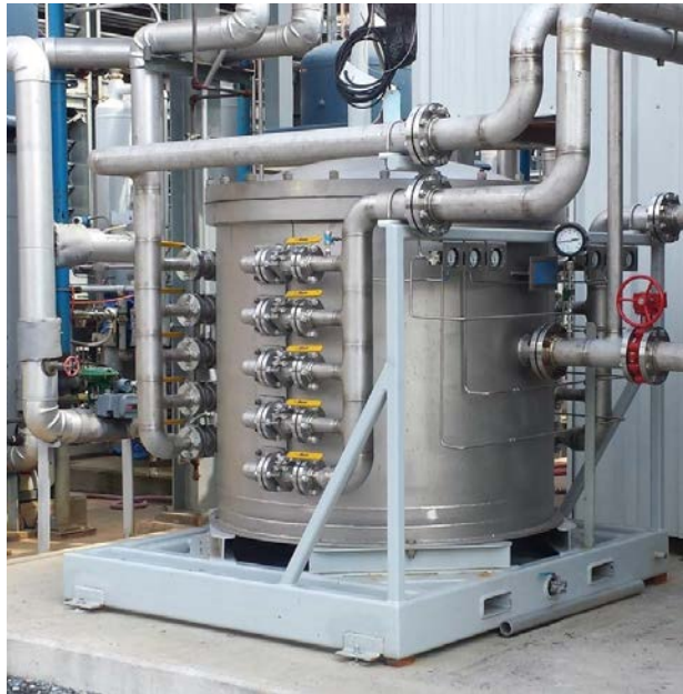
Figure 7: 500-m 2 plate-and-frame module skid
