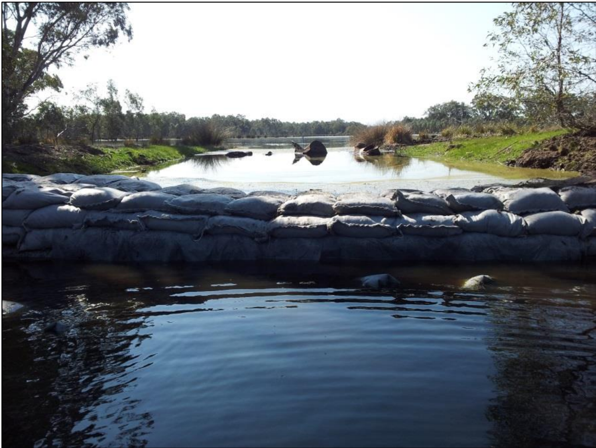
Figure 18 – The 45cm difference in water level upstream (top) and downstream (bottom) of the trial structure – a small but significant margin, with additional depth of water over 60-100 hectares of wetland habitat and re-instatement of natural flows, the trial has had a substantial impact.
