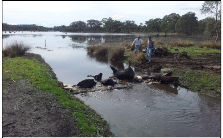
Figure 10 – The First Step – Constructing a hessian sandbag and log bund to reduce flow rate and (to a lesser extent) depth in the channel.
