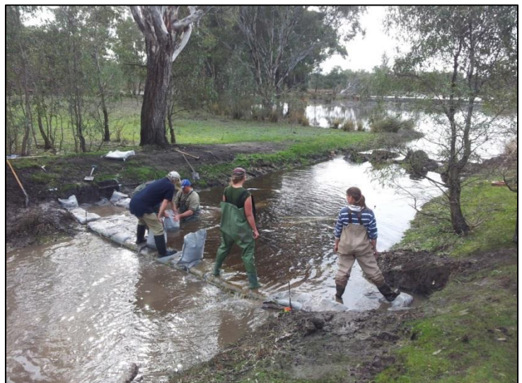
Figure 11 – The sandbag crew succeeding in getting the weir to reach the height of the channel water level. Notice the minor drop in water level downstream as the weir under construction starts to hold back water.
