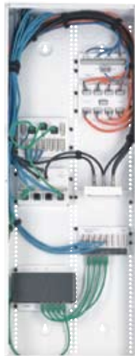
C-0030 Shown Wired (Cover Not Shown - Wires Not Included)
