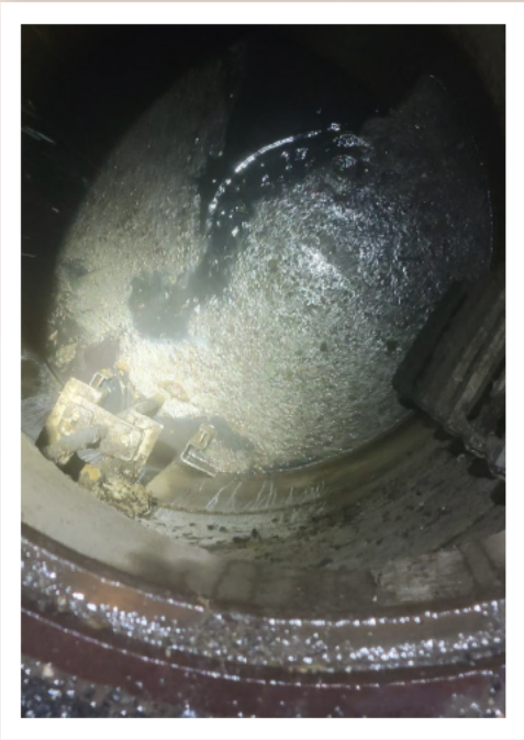
Avenue A Bufferline Clogged manhole over 12 feet deep
