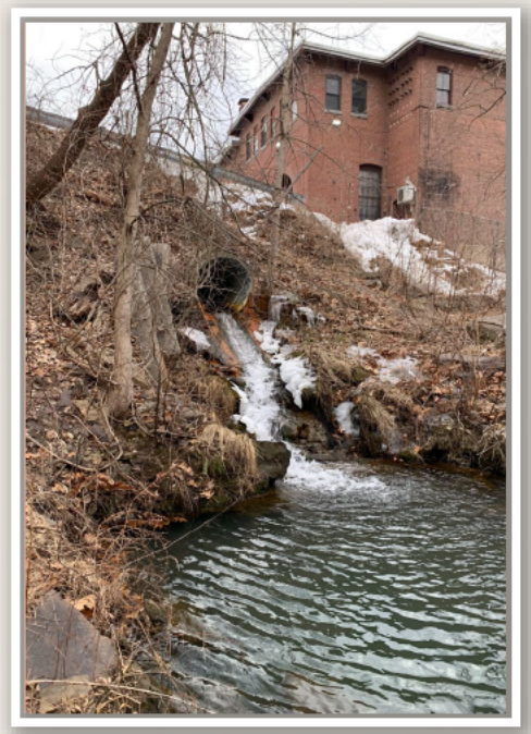
“Dry Weather Discharge”
