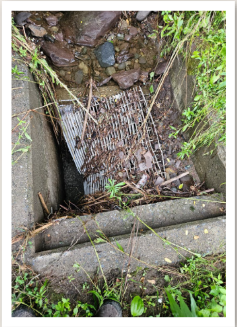
Roadside drainage Damaged, unsafe
