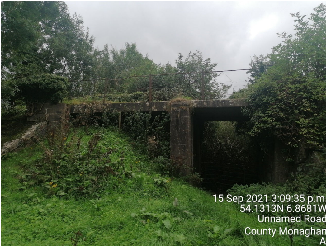
ST13 – Looking West at ST13, the South Span is infilled. The parapet is not suitable. The overgrowth and infill should be removed in the presence of an engineer to assess the structure fully
