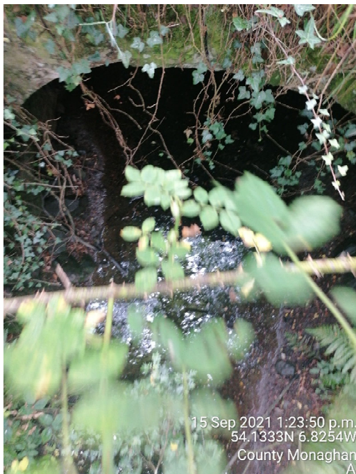
ST12 = Masonry Arch picture taken from the deck. Unprotected steep edge and overgrowth prevent access.
