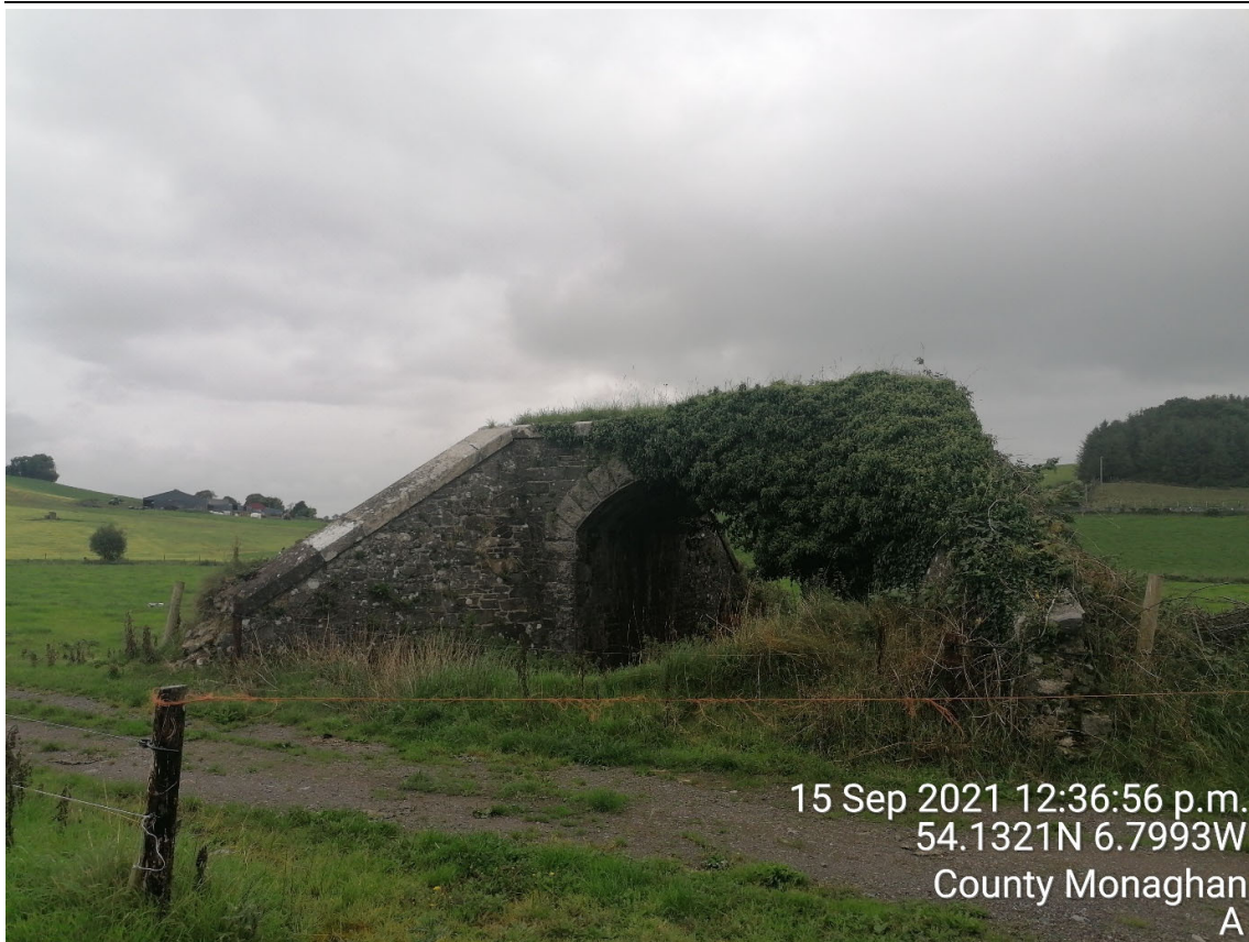
ST11 – Masonry structure retained but embankment deconstructed to the East and West.
