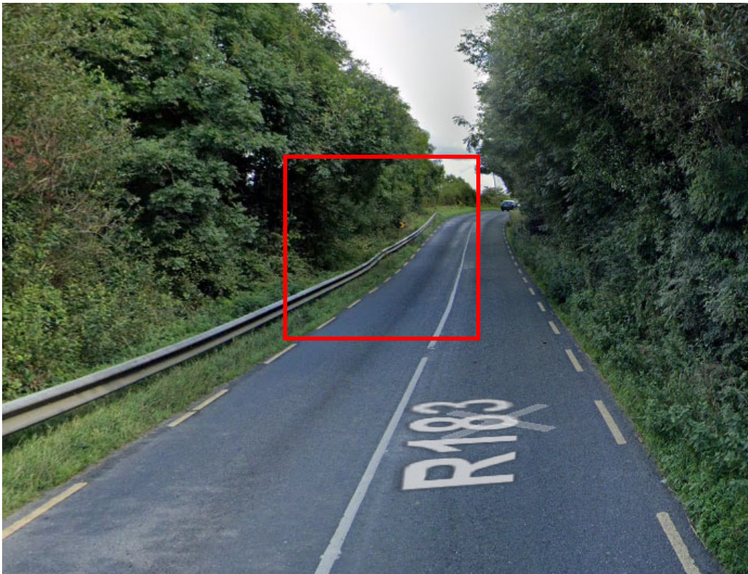
ST07 – Bottom: Damage to VRS is noted.
