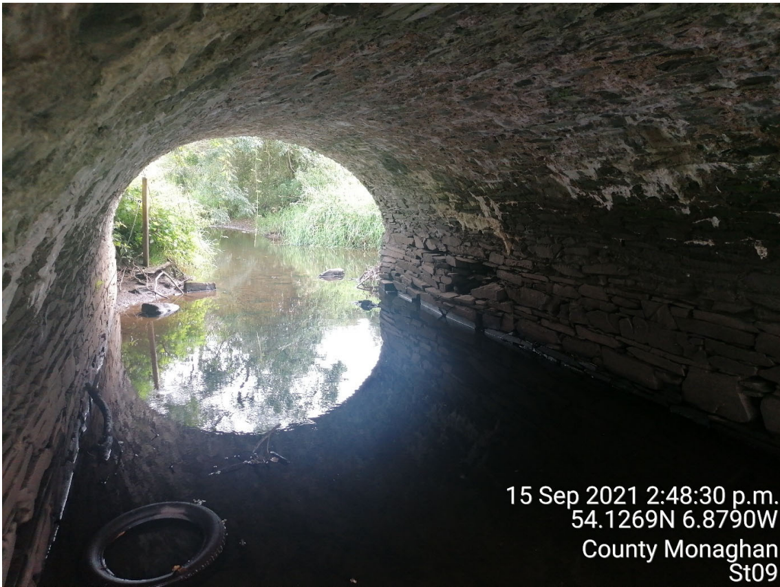
ST09 – Picture looking West under ST09 showing scour issue in South bank
