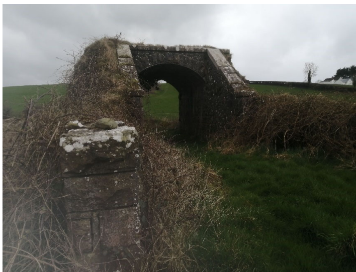
Figure 5: Remnants of Rail Bridge
