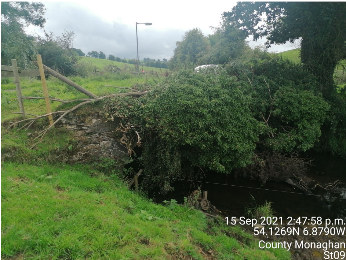
ST09 – Picture looking West at ST09 showing overgrowth and collapsed parapet
