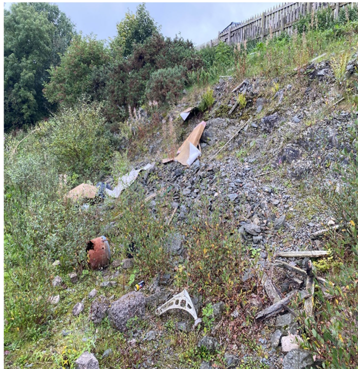
Figure 19: Household waste dumped at embankment behind housing estate at Castleblayney
