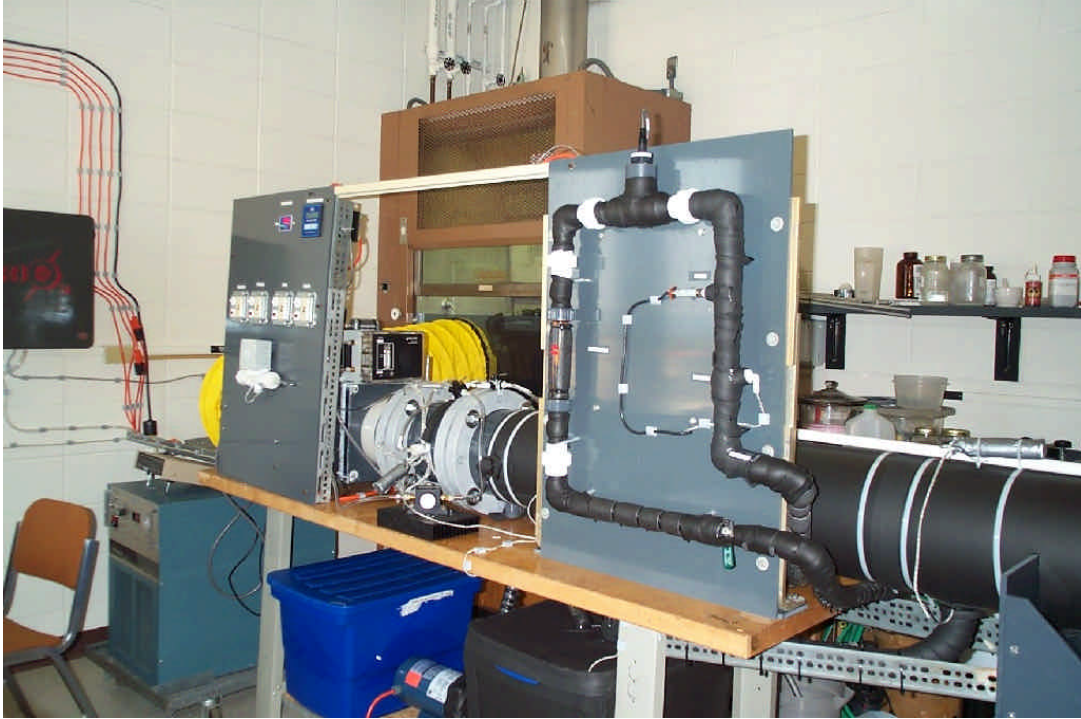
Figure F.3 View on the control panels
