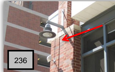
Outdoor WiFi Access Point
