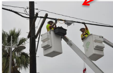
Aerial WiFi Access Point
