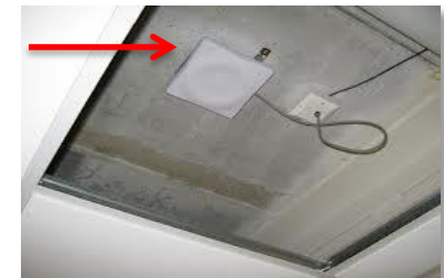
Indoor WiFi Access Point
