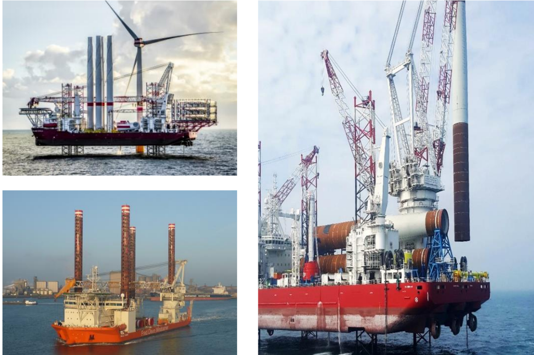
Figure 7. Typical monopile and jacket foundation installation vessels (Figure 3.3-4 of the New England Wind Draft Construction and Operations Plan Volume 1, Epsilon 2021).
