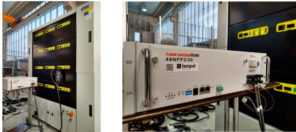
Figure 1. (Left) Laboratory facility for battery testing. (Right) Battery connected to SBT-10050 test equipment.
