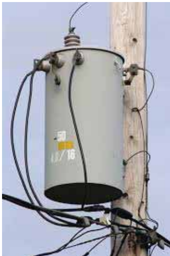
Pole Mount Tx Refurbs
