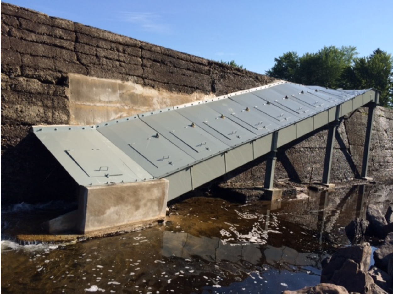
FIGURE 9. PROJECT UPSTREAM EEL PASSAGE FACILITY – ORONO PROJECT
