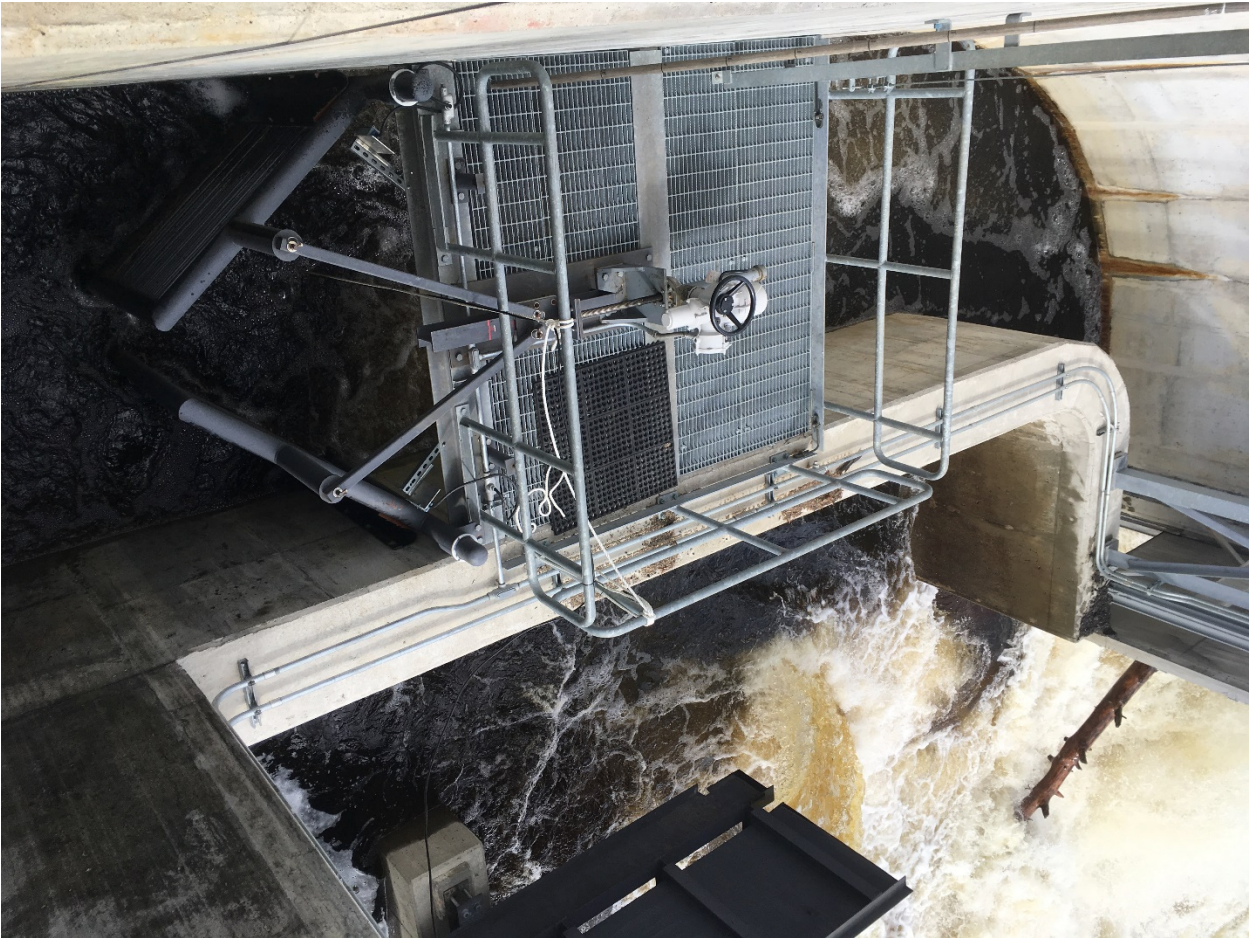
FIGURE 8. PROJECT FISH LIFT AND TRAP FACILITY – ORONO PROJECT
