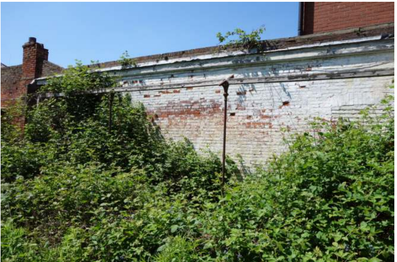
4.20: Ruinous lean-to arcade
