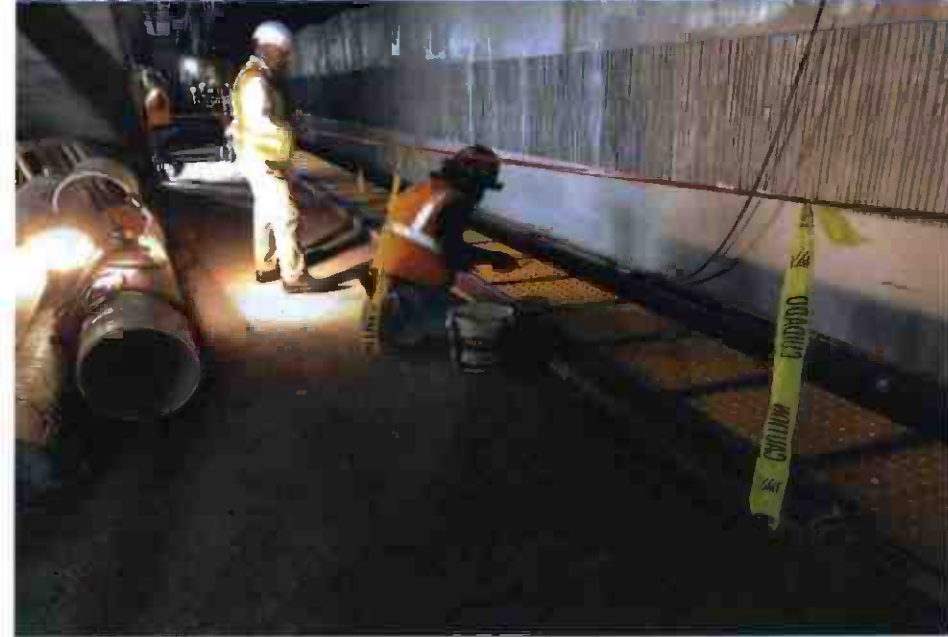
Vernon Station – Continued installation of edge pavers on the north and south bound platform level
