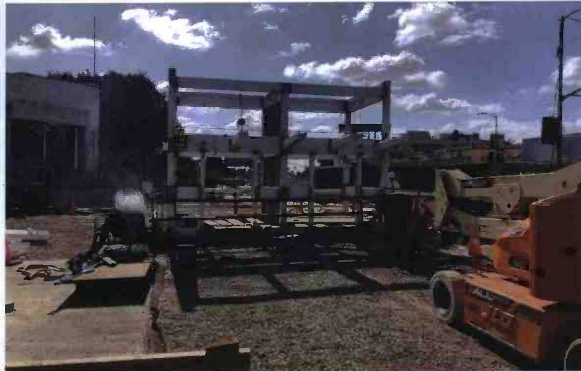
Leimert Park Station – Continued installation of entrance canopy steel for elevators 1 and 2 at the plaza level
