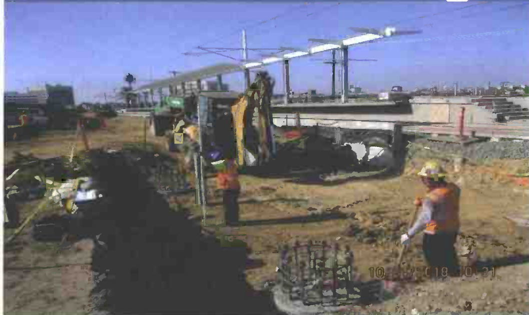
Grading for grade beam and slab at the La Brea Station east fare gate
