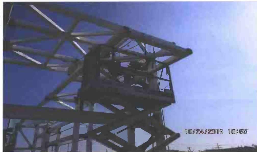
Welding brackets and plates in process at the east fare gate at the Fairview/Heights Station
