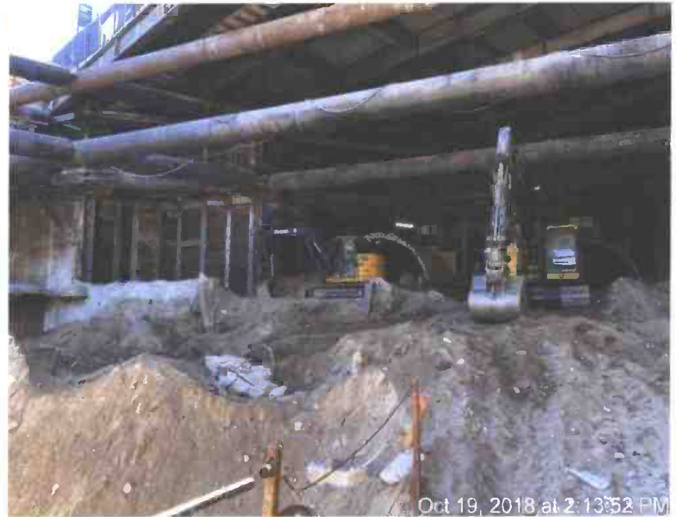
Oct 19, 2018 at 2:13:52 PM Excavation/lagging and removal of tunnel segments under Central decking
