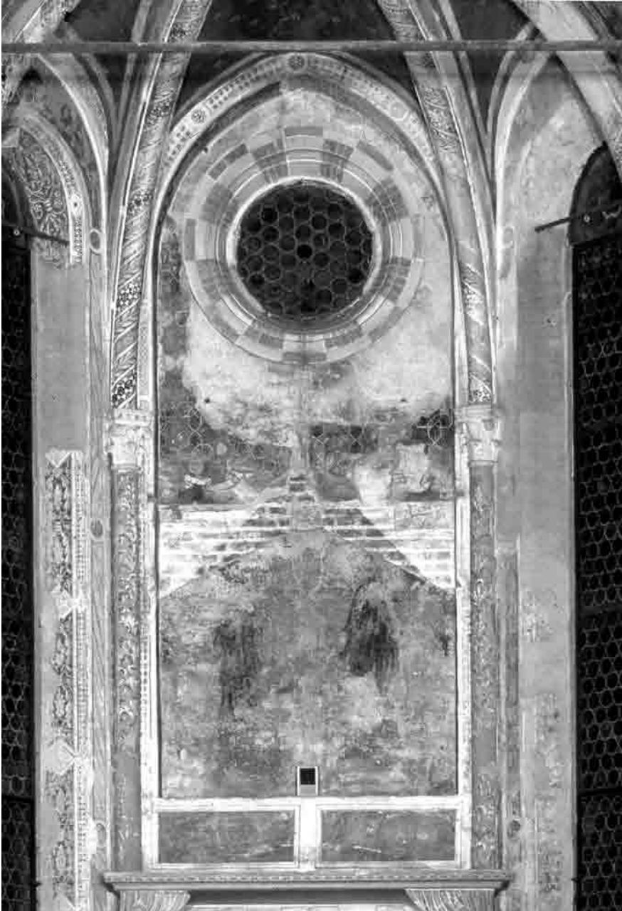
Fig. 7. Central bay of apse, east end of Arena Chapel, Padua, detail of blind bay with oculus, traces of canopies, frescoed drapery, and box-shaped ledge directly above later tomb shown in fig. 4. Private photo collection.
