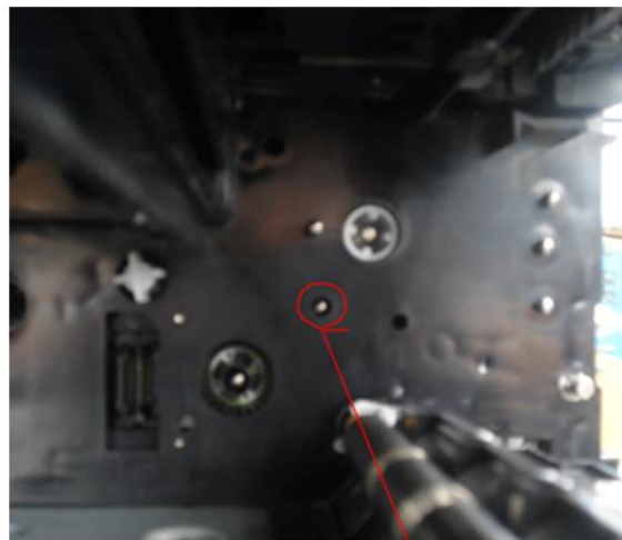
Frame main's cleaning & checking point
