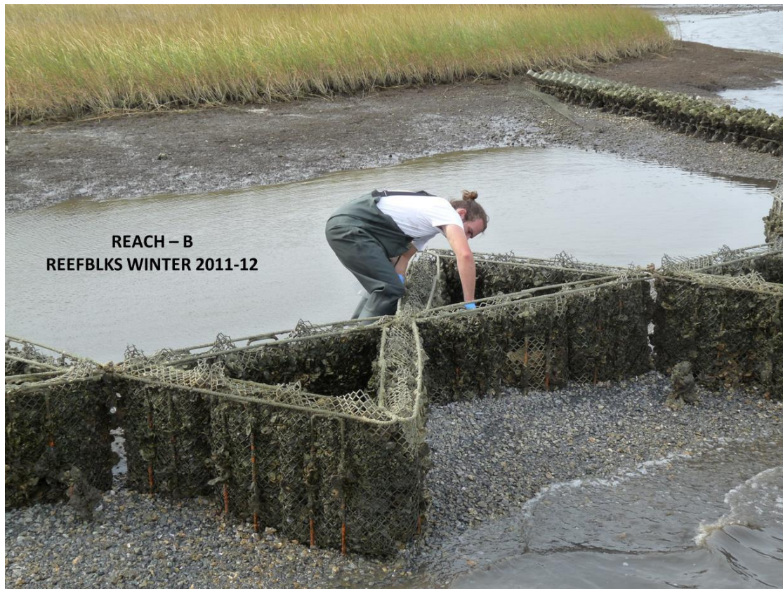
Figure 45. Photo of Reach B ReefBlks at low tide during the winter 2011-12 assessment, showing successful colonization. Also notice the shell and limestone on the bottom of the windward side. A-Jacks used to tie-in the flank of the project are seen in the background.
