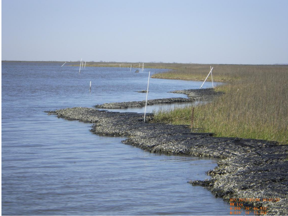
Photo 13: View of Gabion Mats low area and transition to ReefBlks on Reach E looking north
