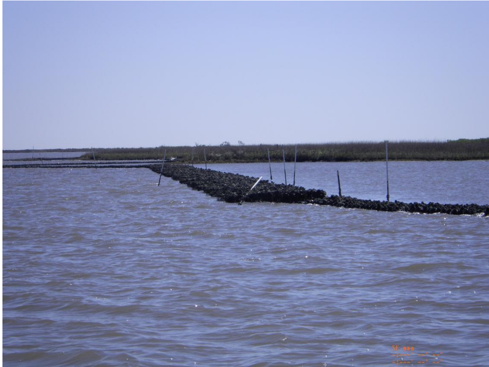
Photo 9: Transition of ReefBlks to the shoreline tie-in on north side of Reach B
