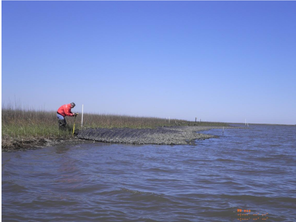
Photo 5: Gation Mats located on the southern end of Reach B looking north
