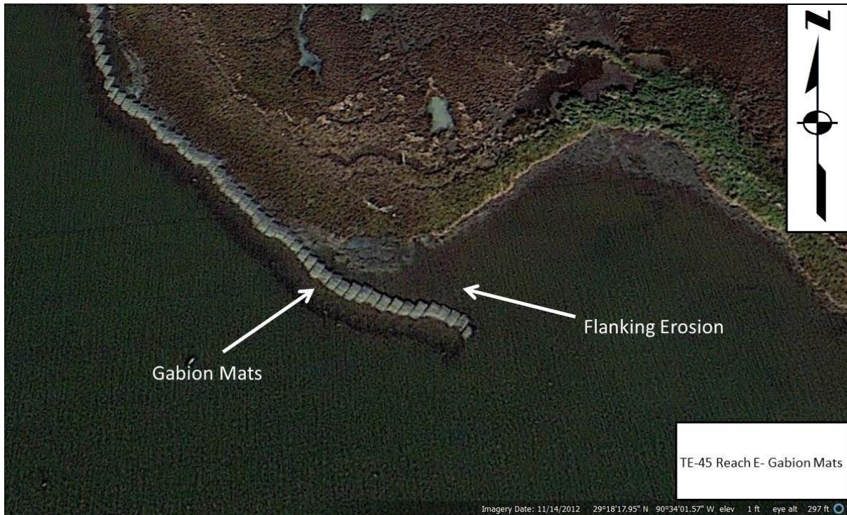
Figure 18. November 14, 2012 image depicting flanking erosion behind the Reach E Gabion Mat treatment at the Terrebonne Bay Shore Protection Demonstration (TE-45) project. Image reproduced from Google Earth.
