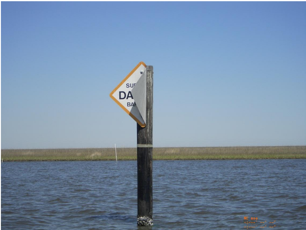
Photo 18: View of Damaged warning sign along Reach E
