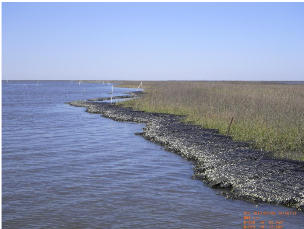
Photo 12: View of Gabion Mats on the south end of Reach E looking north
