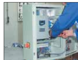
Controle paneel met frequentie omzetter Control panel with frequency inverter
