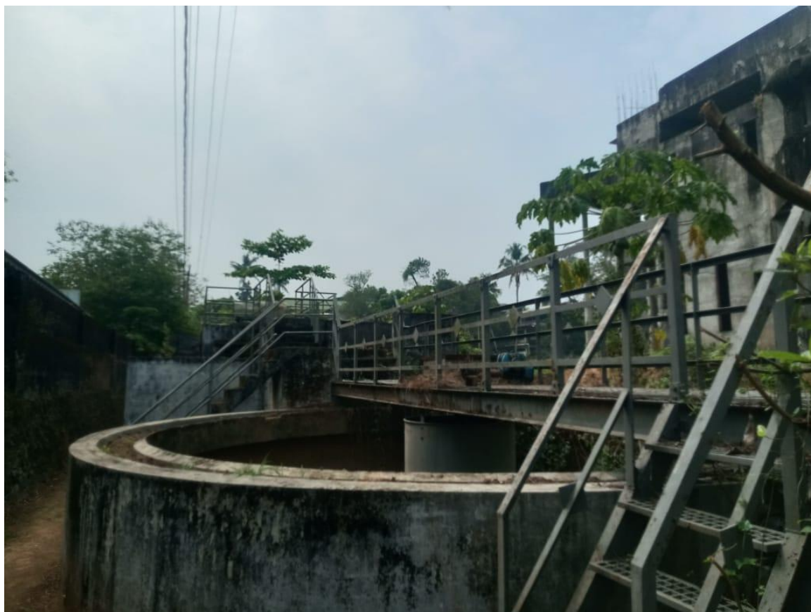
Fig.2.2 Existing Storm Water Treatment Plant at Aluva
