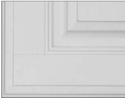
Example of door front joint separation
