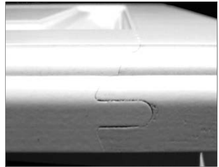
Example of door end joint separation
