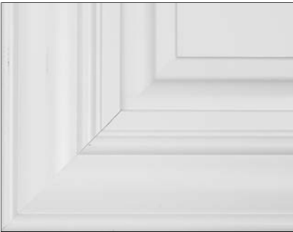
Example of door front joint separation
