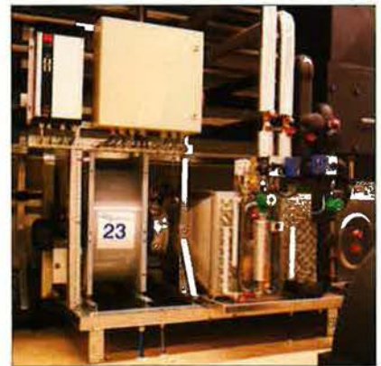
air-handling systems for mushroom growing.
