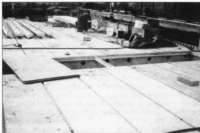
Figure 6. Nozzle floor with grooves for cleaning.
