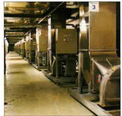
air-handling systems for phase 1, 2 and 3 tunnel composting.
