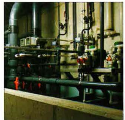
air-scrubbers, air-washers and biofilters.
