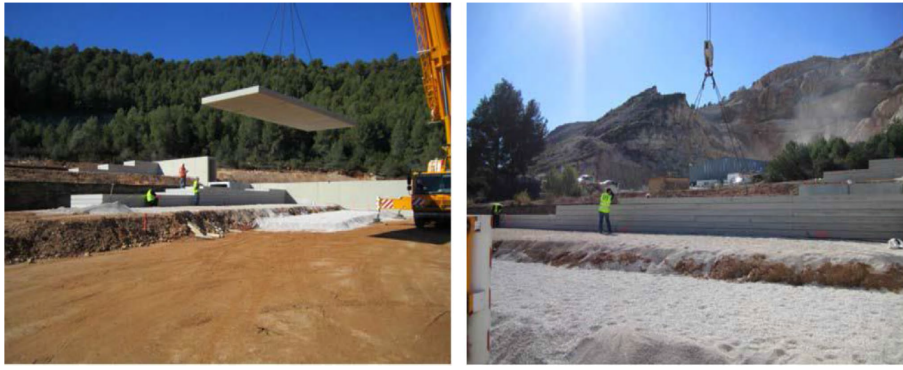
Figure 3: Installation of the prefabricated and granular wedge in a stone quarry located in Oliva (Valencia) Spain
