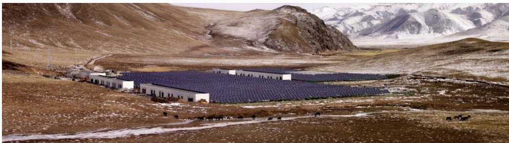
2 MW Utility-scale PV in Yushu, Qinghai Province, China, Courtesy of Lu Fang
