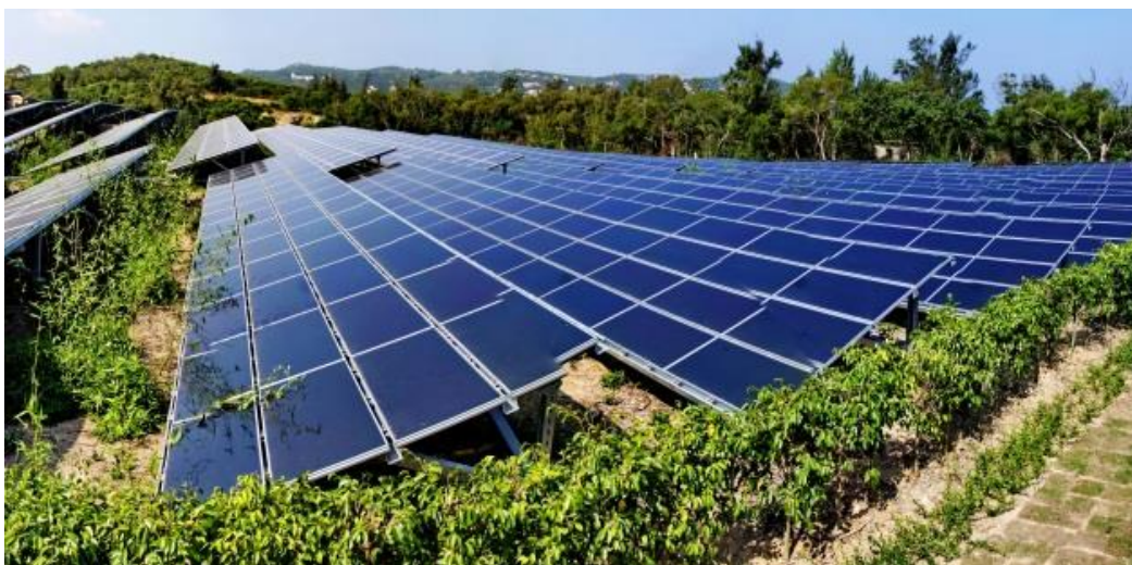
600 kW PV, Donggao Island, Guangdong, China, Courtesy of Lu Fang
