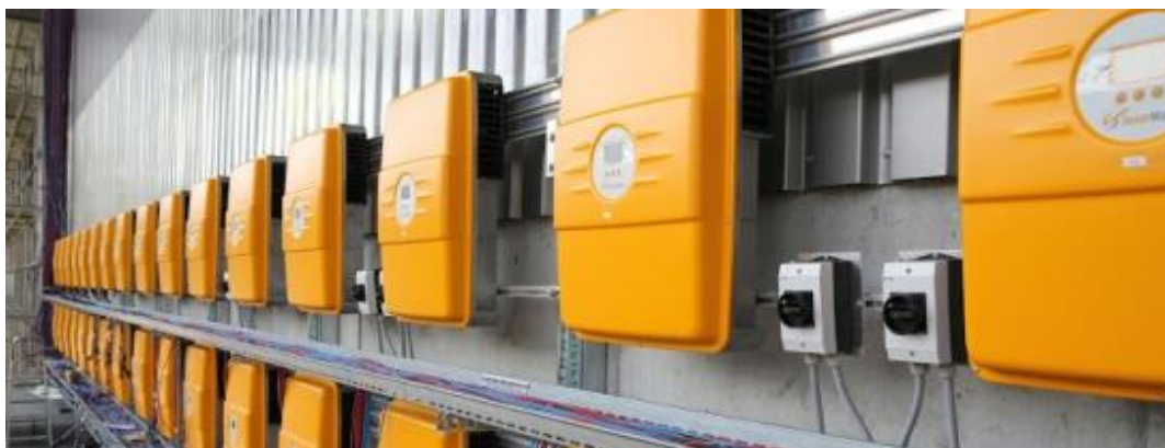
Inverters at a 555 kW commercial PV plant, Kölliken, Switzerland – Courtesy of EcoenergieA+, Schöftland, Switzerland
