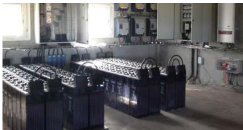
AC coupled PV/Diesel/Batteries Hybrid system implemented at Isona (Lerida), Spain by Granjes Pereto
