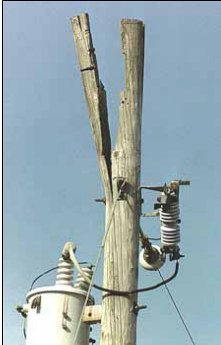
Figure 6 (Photo 05B15) Badly split pole top, Circuit V79594, northwest of Barrow
