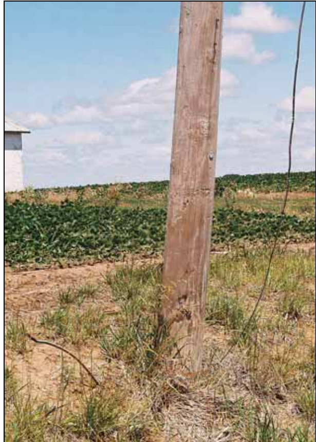
Figure 25 (Photo 05P5) Broken ground wire & ground rod partially pulled out of ground, Cir. U04538, CH 9C, south of Pleasant Plains
