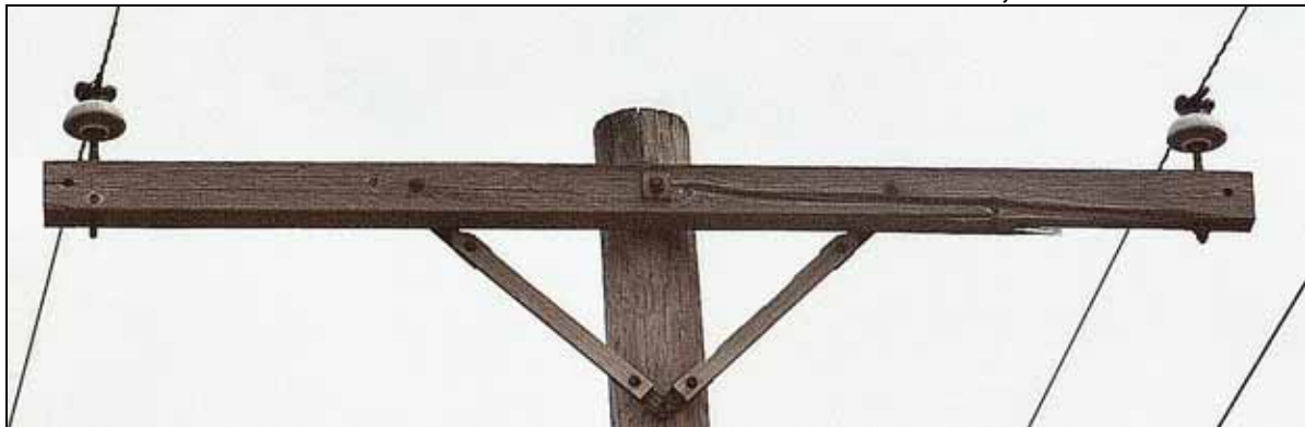
Figure 10 (Photo 05D5) Split crossarm, Cir. X96543, S. of Lawrenceville
