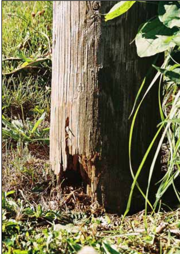
Figure 24 (Photo 05P1) Pole damaged at ground line, Circuit U04538, Main St. east of Jackson St., Pleasant Plains
