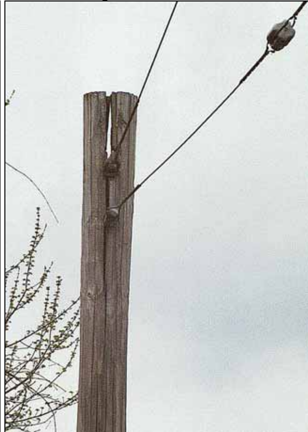
Figure 13 (Photo 05D18) Guy stub pole badly split at top, Circuit X96543, 9 th & Meagher Sts., St. Francisville
