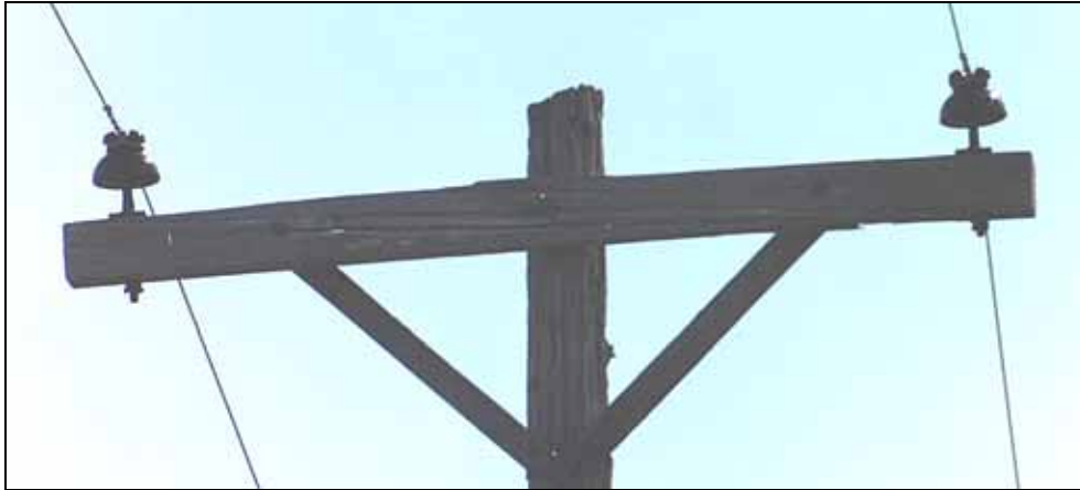
Figure 4 (Photo 05B10) Split & deteriorated crossarm and badly shell rotted pole, Circuit U39541, southeast of Golden
