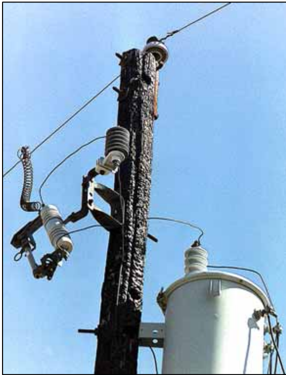
Figure 2 (Photo 05B3) Burned pole top (lightning damaged?), Circuit U39541, Main & Maple Sts., Timewell
