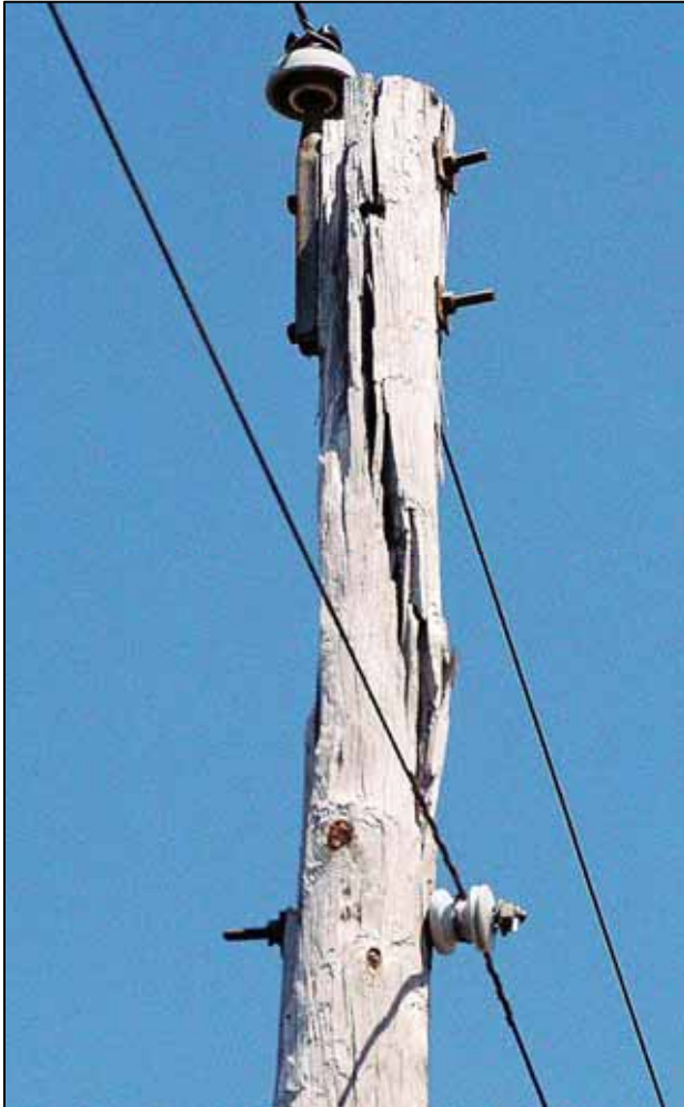
Figure 21 (Photo 05K8) Lightning damaged pole top, Circuit Y60593, Road 2800N, east of Rantoul
