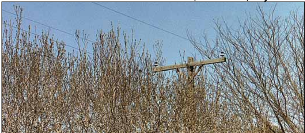
Figure 3 (Photo 05B6) Trees into primary, Circuit U39541, Madison St., Clayton
