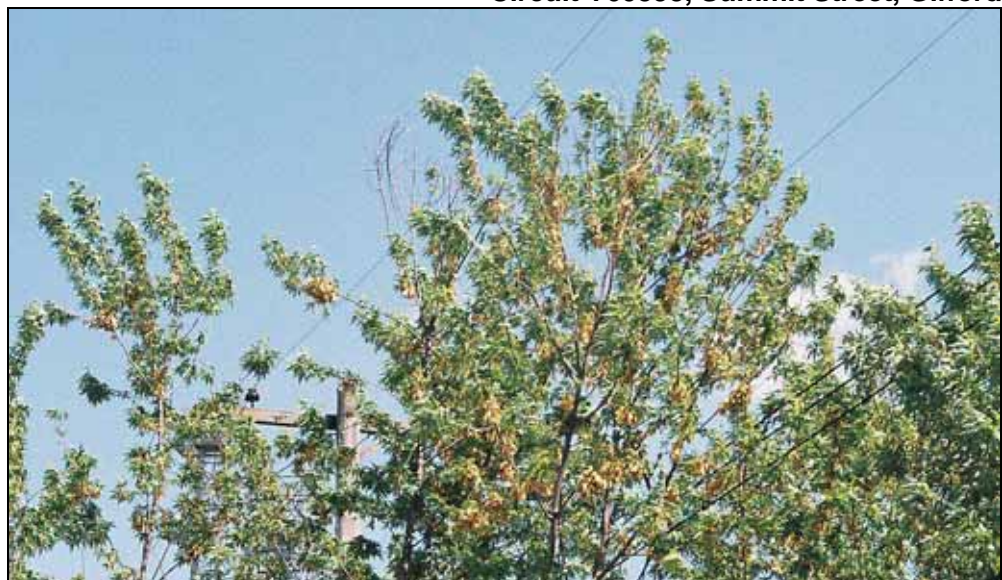
Figure 23 (Photo 05K9) Soft maple tree into primary, Circuit Y60593, Summit Street, Gifford
