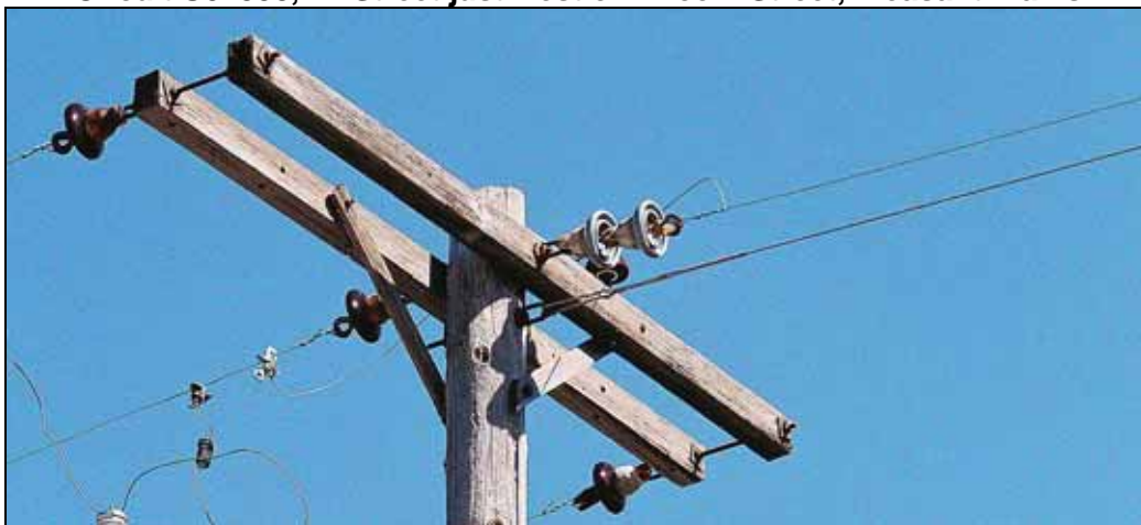
Figure 27 (Photo 05P4) Overhead guy wire deadended 6" to 9" below 7.2 kV primary conductor on same pole, (NESC clearance violation--12" minimum clearance required) Circuit U04538, 4 th Street just west of Lincoln Street, Pleasant Plains
