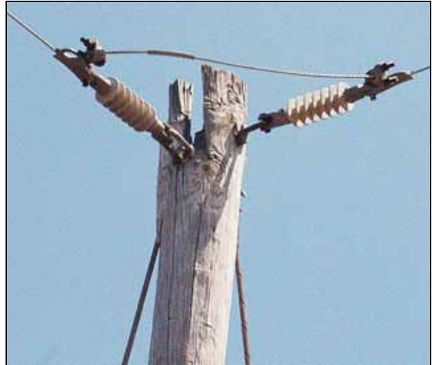
Figure 22 (Photo 05K7) Badly split pole top, Circuit Y60593, east of Rantoul
