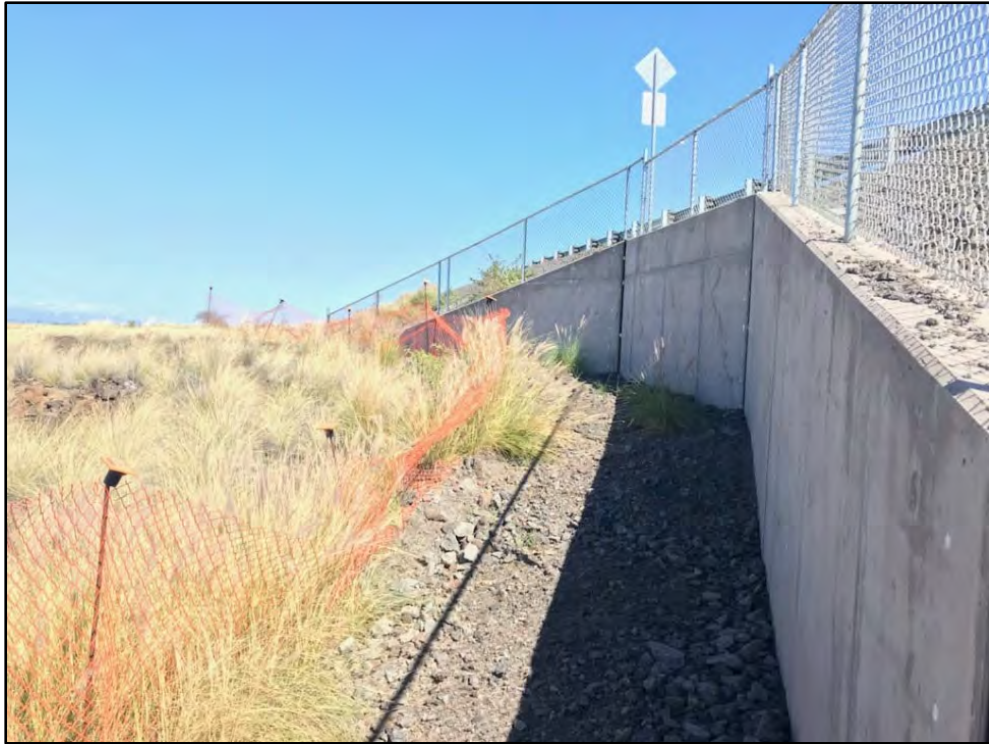
Figure 48. Photo of the northern section of Retaining Wall G; view to north
