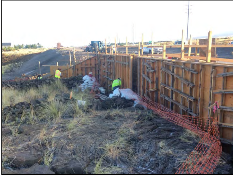
Figure 52. Photo showing construction of concrete forms for Retaining Wall F; view to north
