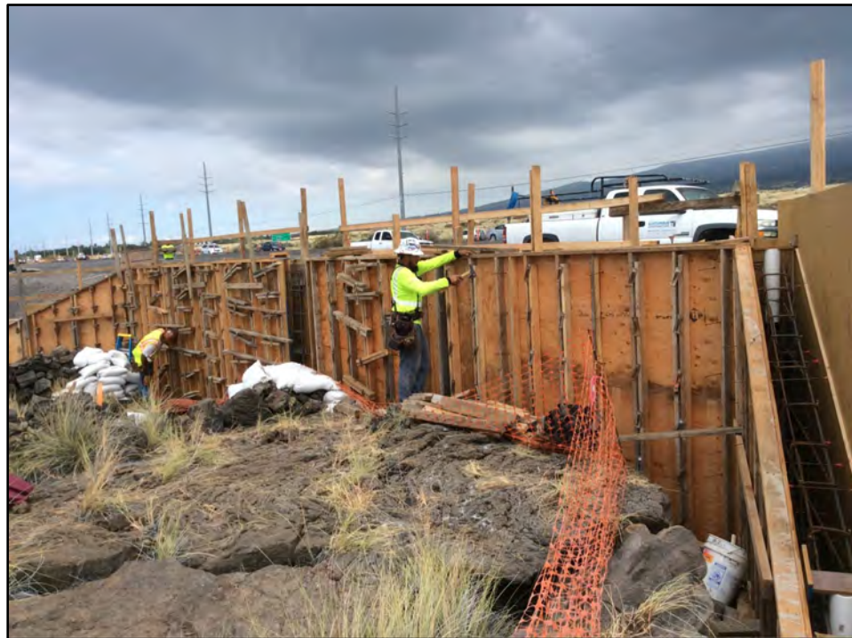
Figure 53. Photo of workers constructing the wooden concrete form for Retaining Wall F; view to north
