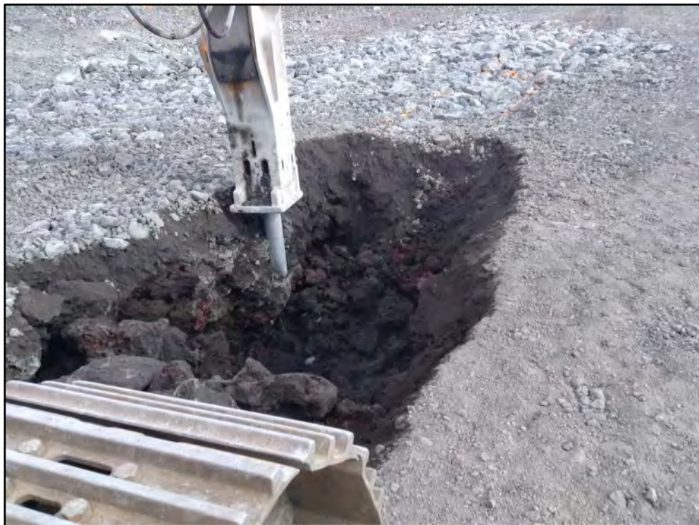
Figure 57. Photo of Lava Tube Breach #1 being collapsed by an excavator; view to northwest
