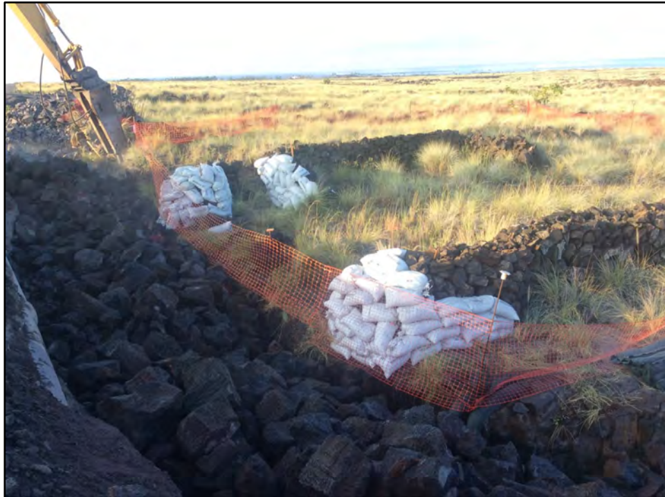
Figure 51. Photo of SIHP #s -10154 and -06432 with supportive sandbags in place; view to southwest
