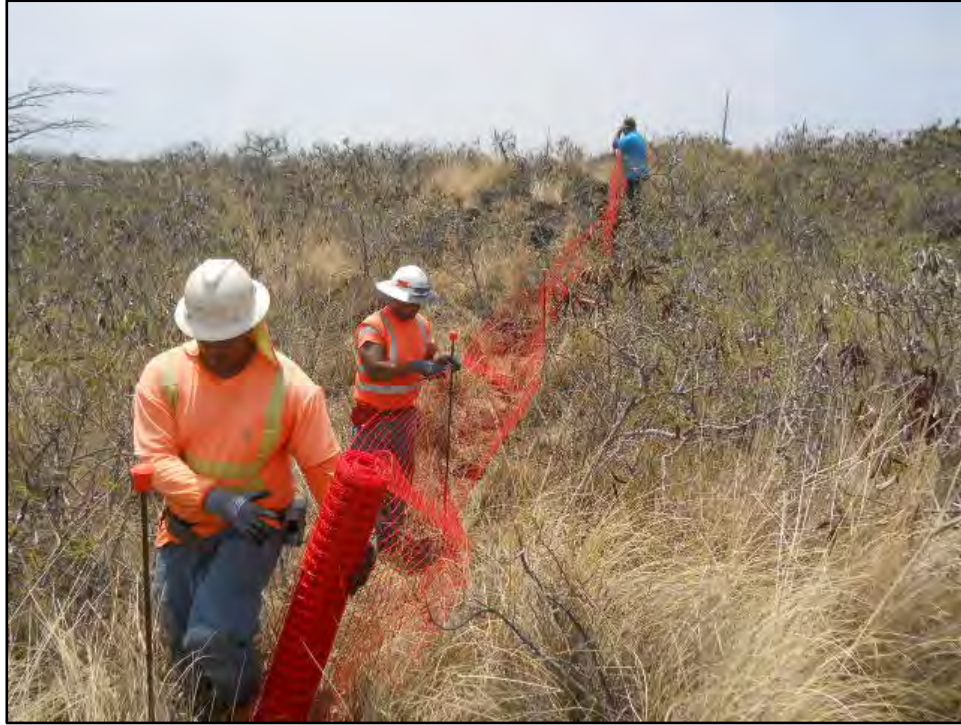
Figure 37. Photo of GBI crew installing fencing at SIHP # -19950 on 1 June 2015; view to north
