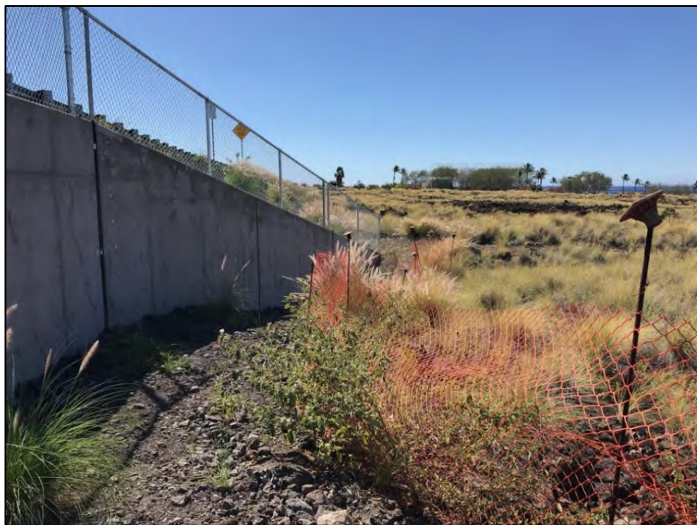
Figure 49. Photo of the southern section of Retaining Wall G; view to southwest
