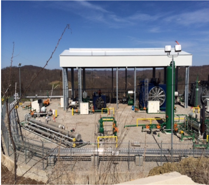
Figure 7-2: UNG Compressor Station
