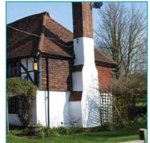
Simple plain hanging tiles found on the gable to Barcombe Farm House
