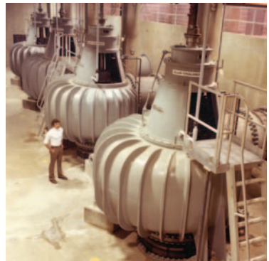
54" WSYV pumps in primary influent service. Each pump rated for 69,500 gpm.
