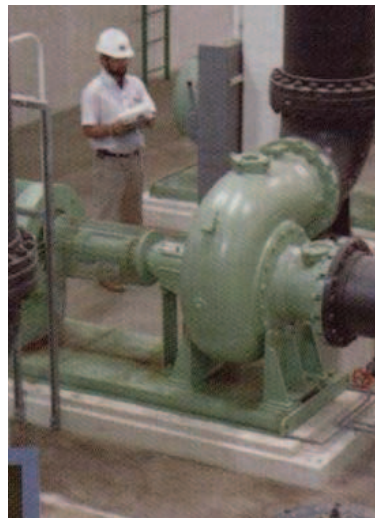
16" NSY unit on digester service.
