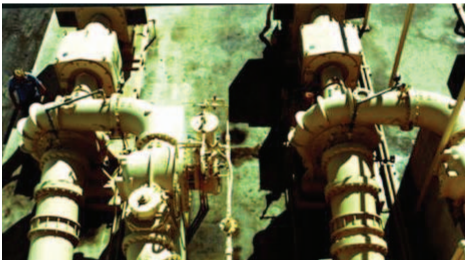
24" Model NSSE pumps handling wastewater in Florida.
