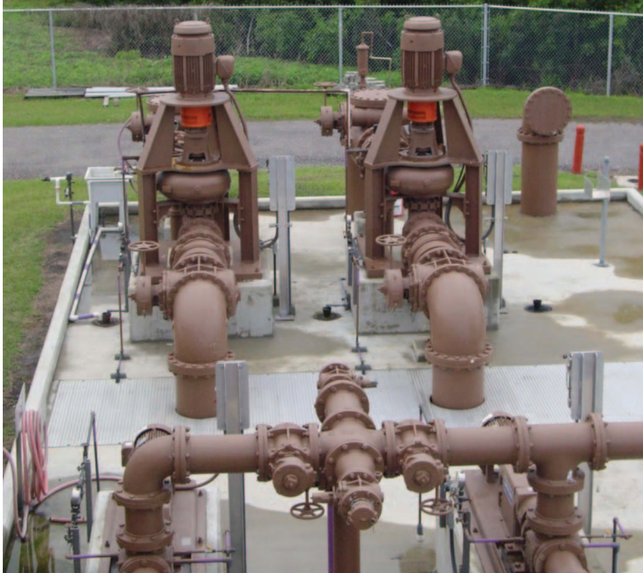
Model NSWV pumps with PEG base installed in a sewage treatment plant in Florida.
