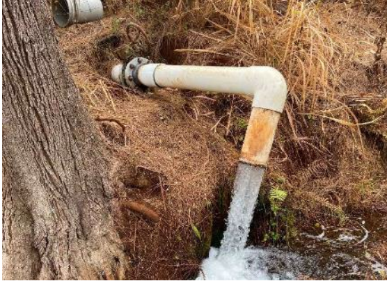
A) Water was originally released from a valved pipe from Reservoir 1 into the South Waikapū ‘Auwai, experiencing high amounts of water loss.
