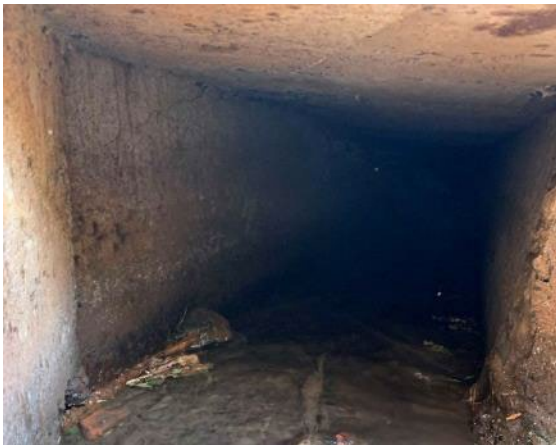
C) Water flows in an underground concrete-lined channel behind Wailuku Public Library.
