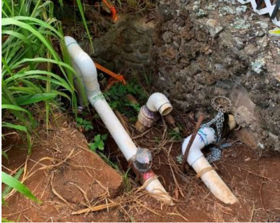
A) Distribution pipe with valve chained and flow meter at center, located on the boundary of Imua Family Services property.
