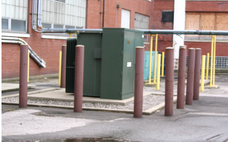
Photo 4: View of the transformer located in the open lot behind Century Centre I.
