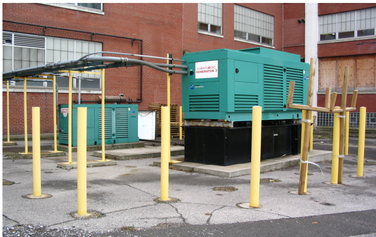
Photo 3: View of the generators located in the open lot behind Century Centre I.
