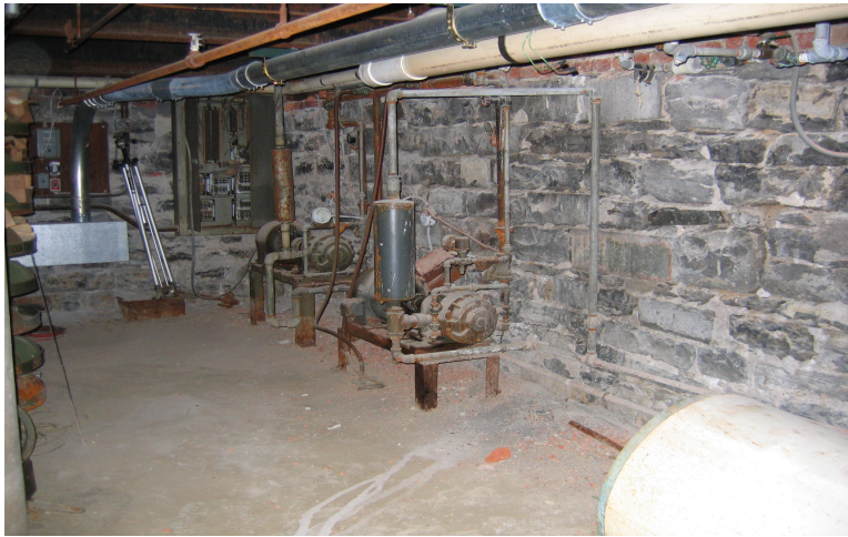
Photo 8: View of one of the older mechanical systems located in the basement of Century Centre I. No spills or leaks were identified in the basement.
