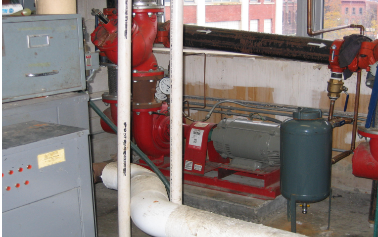
Photo 13: View of one of the typical mechanical rooms located on the 3 rd and 4 th floor of Century Centre I. The transformers located throughout the building are dry type transformers and do not contain PCBs.
