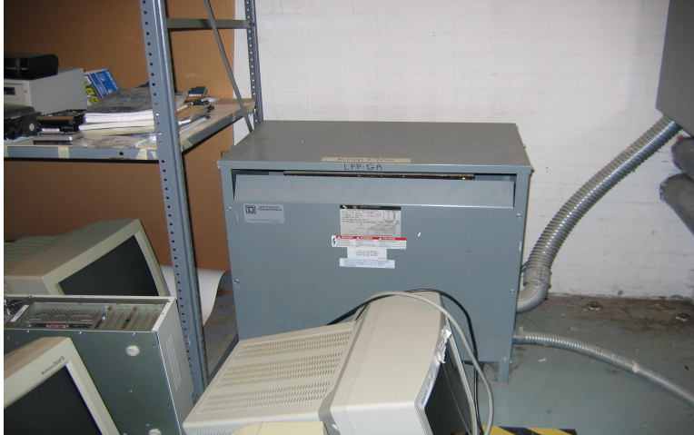
Photo 7: View of one of the dry transformers located throughout the building.
