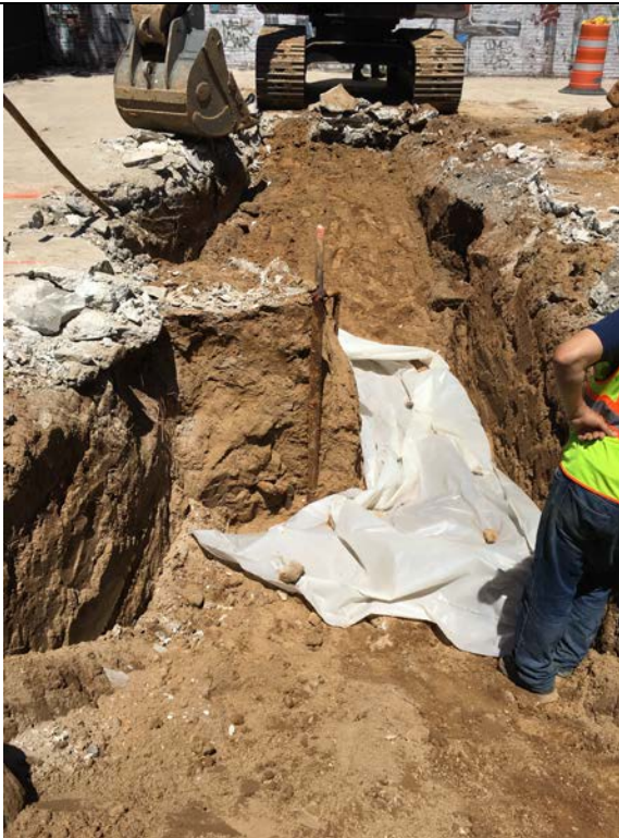
Photo 27: Demarcation layer (i.e. polyethylene sheeting) placed on top of the USTs. Photo taken June 26, 2017.
