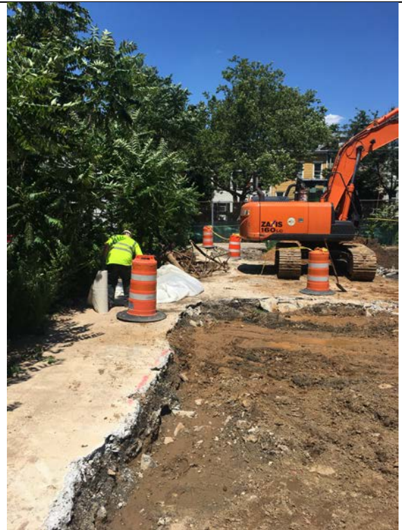
Photo 16: Stockpiled contaminated soil along western portion of Site. Photo taken June 20, 2017.
