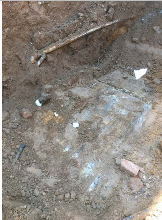
Photo 20: Underground storage tank (UST) identified in Trench 6. Photo taken June 22, 2017.
