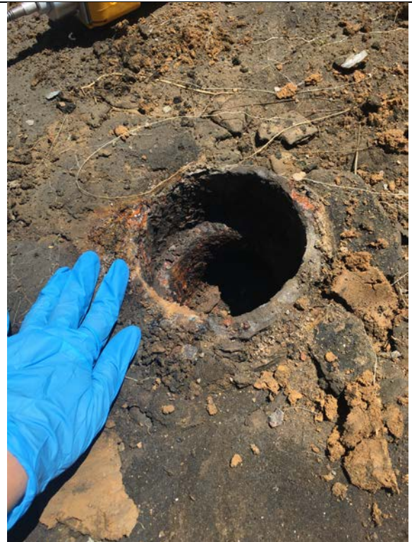
Photo 12: 6-inch diameter vertical pipe associated with the drain identified on the feature in Trench 2. Photo taken June 20, 2017.
