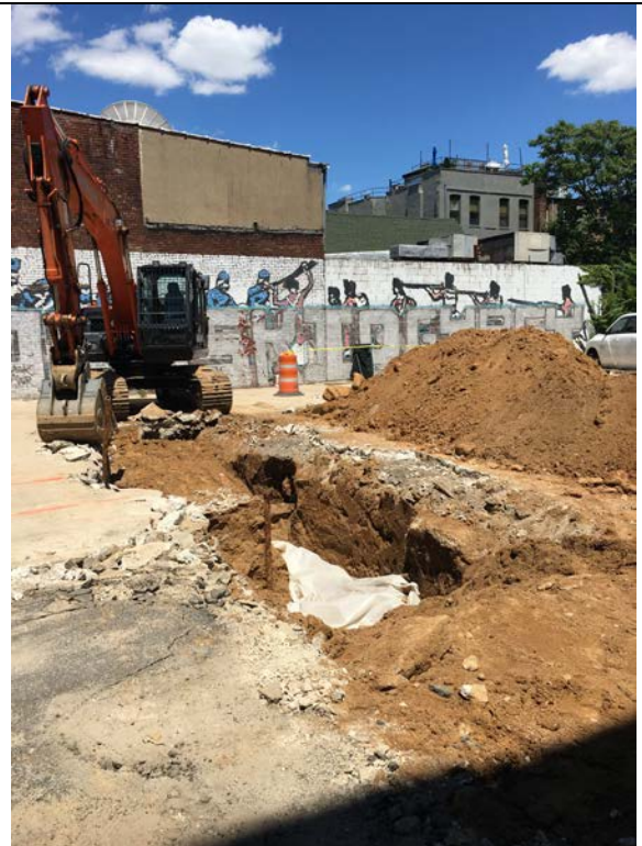
Photo 28: Additional view of demarcation layer (i.e. polyethylene sheeting) placed on top of the USTs. Photo taken June 26, 2017.
