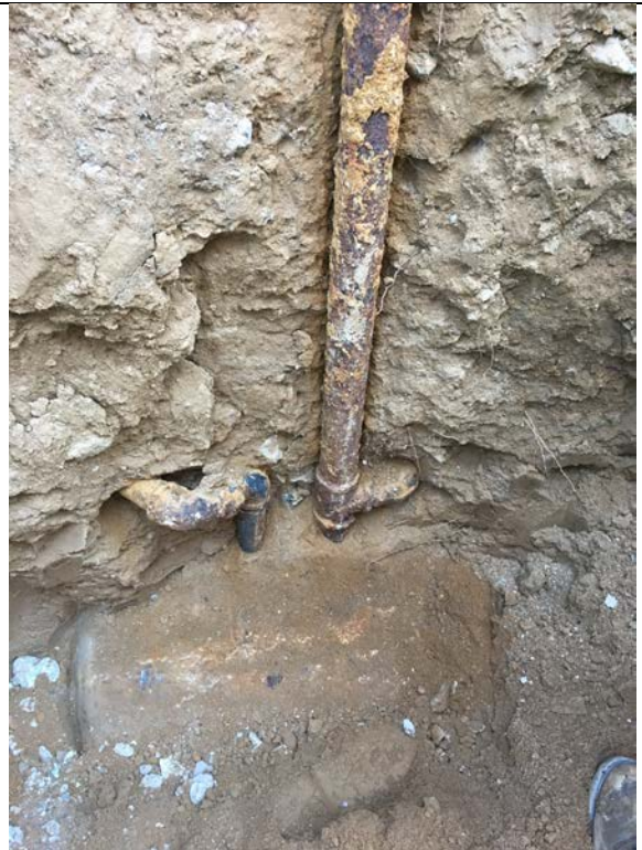
Photo 24: One of two steel underground storage tanks (USTs) identified in Trench 8. Photo taken June 26, 2017.
