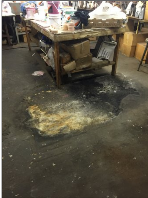
Staining observed within interior of plastic manufacturing facility.
