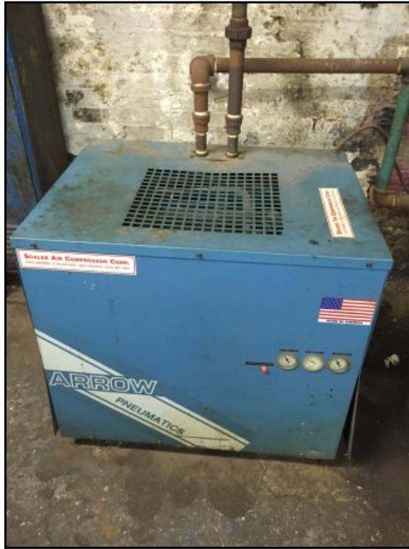
Machinery located within plastic manufacturing facility.
