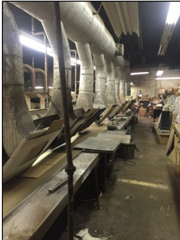
Vent hoods associated with painting
