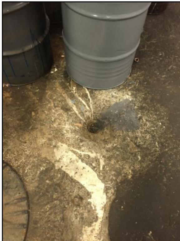
Staining observed entering floor drain within interior of plastic manufacturing facility.
